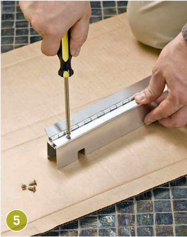
Working on the floor or another flat surface , attach the door hinge to the hinge jamb, if required. In most systems, the hinge is fitted over the hinge jamb after you attach it to the wall.
