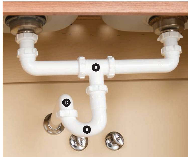
A "center tee" arrangement has a single P-trap (A) that is connected to a waste tee (B) and the trap arm (C).
