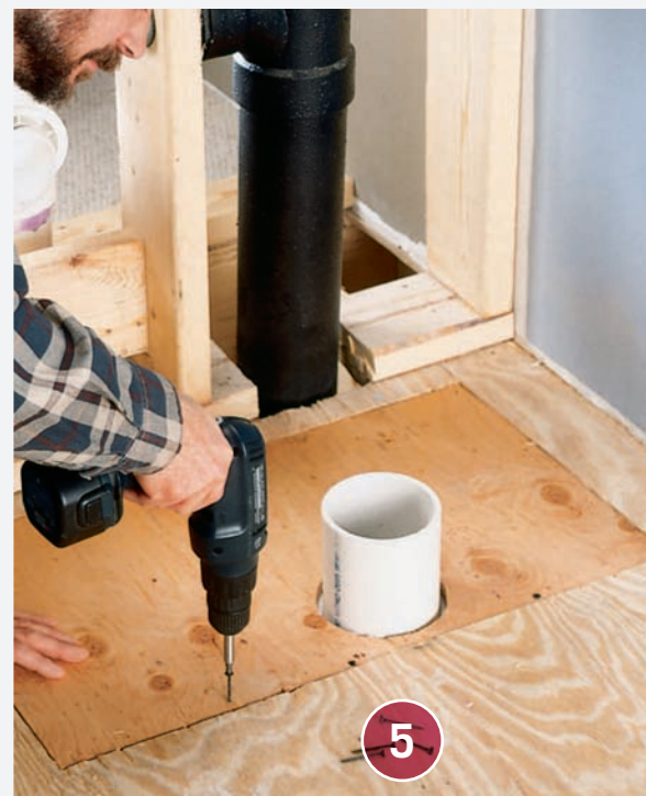
Cut a piece of exterior-grade plywood to fit the cutout floor area, and use a jigsaw to cut an opening for the toilet drain stub-out. Position the plywood, and attach it to joists and blocking with 2" screws.
