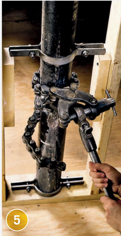
5 Tighten the chain and snap the pipe according to the tool manufacturer's directions.
