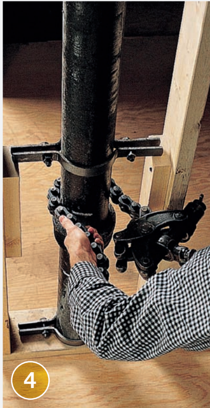
4 Wrap the chain of the snap cutter around the pipe, so that the cutting wheels are against the chalkline.
