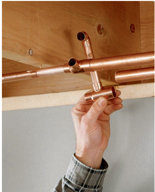
Dry-fit as much of the new line as you can , whether the new pipes are copper or cpvc. Dry-fitting almost always yields more reliable results for DIYers than taking measurements as you go.
