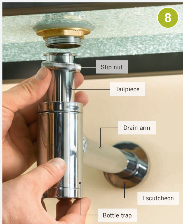
8 Install the bottle trap. Loosen the rings on the top and outlet of the bottle trap. Slide the drum trap top hole over the tailpiece. Slide the drain arm into the side outlet, with the flat side of the rubber gasket facing away from the trap. Insert the drain arm into the wall outlet. Hand tighten the rings.
