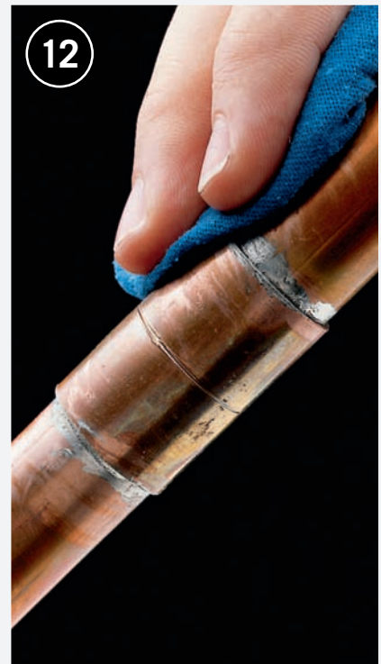
12 Allow the joint to cool briefly, then wipe away excess solder with a dry rag.
