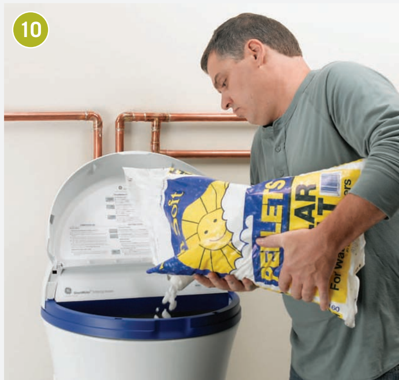
10 Turn on the water supply and make sure the installation works properly. If you see any leaks, fix them. Then add the water softening pellets to the top of the unit in the ratios explained on the package.
