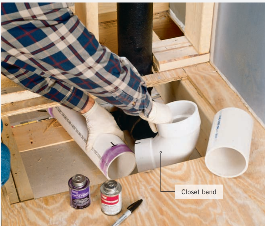
Create a new toilet drain running to the drainage stack , using a closet bend and a straight length of pipe. Position the drain so there will be at least 15" of space between the center of the bowl and side wall surfaces when the toilet is installed. Make sure the drain slopes at least \frac{1}{4} " per ft. toward the stack, then support the pipe with plastic pipe strap attached to framing members. Insert a 6" length of pipe in the top inlet of the closet bend; once the new drain pipes have been tested, this pipe will be cut off with a handsaw and fitted with a toilet flange.
