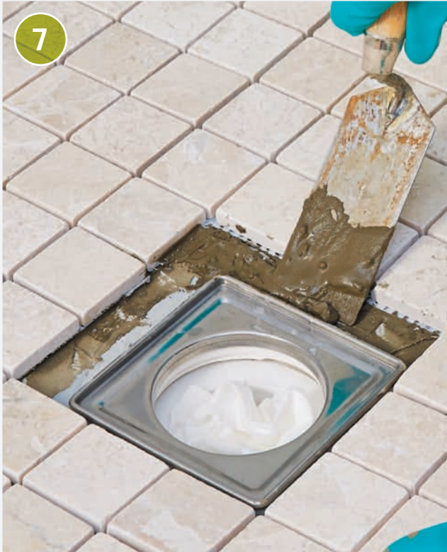
7 Apply thinset onto the shower pan, taking care not to get any on the drain grate mounting plate. You may need to use a small trowel or a putty knife to get into small gaps.
