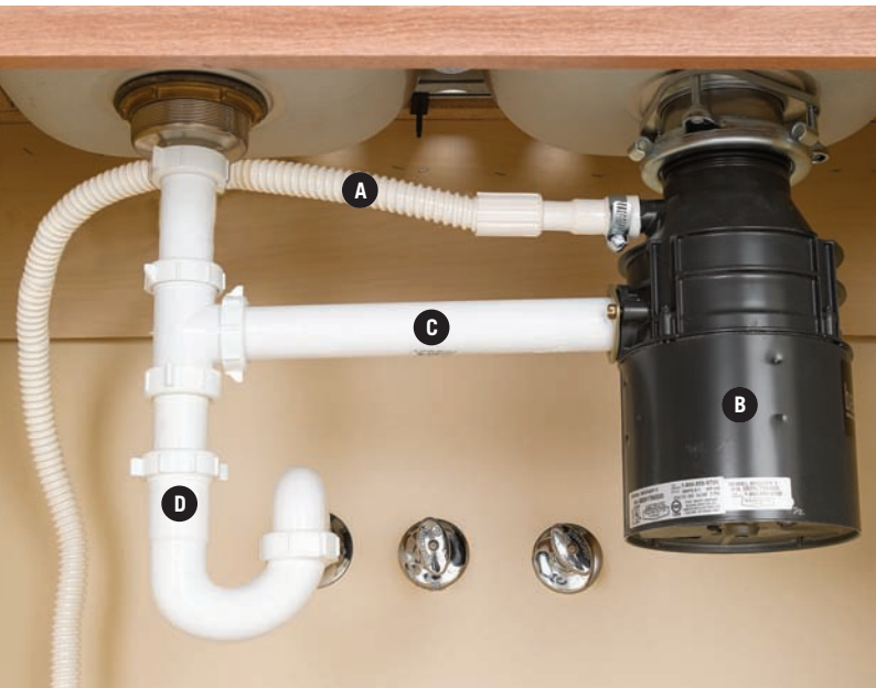
In this arrangement, the dishwasher drain hose (A) attaches to the food disposer (B), and a trap arm (C) leads from the disposer to the P-trap (D).
