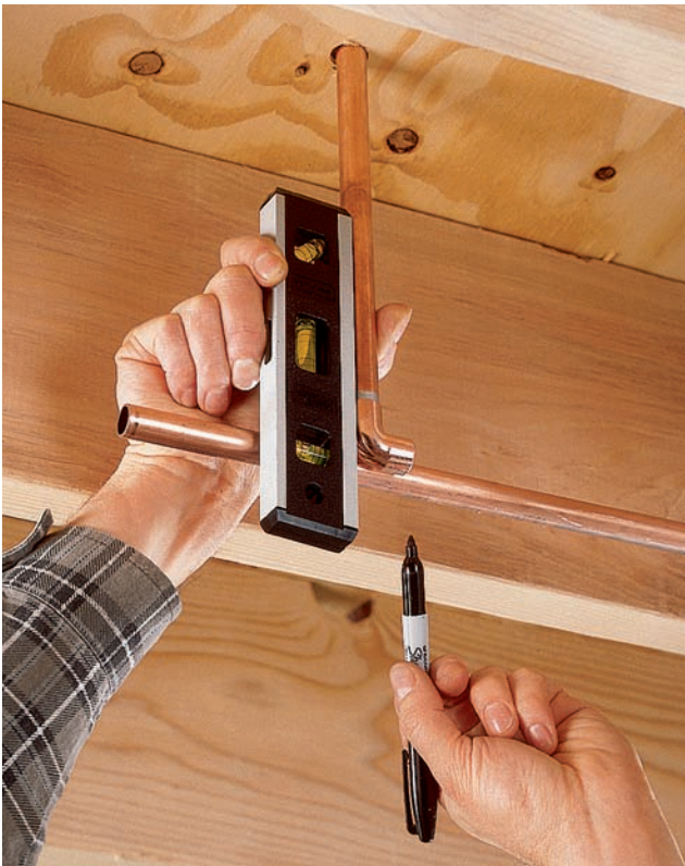
Use a small level to make sure unattached riser pipes are plumb when marking cutting lines on mating horizontal branch lines.
