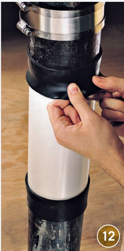
12 Roll the ends of the neoprene sleeves over the ends of the new plastic pipe.
