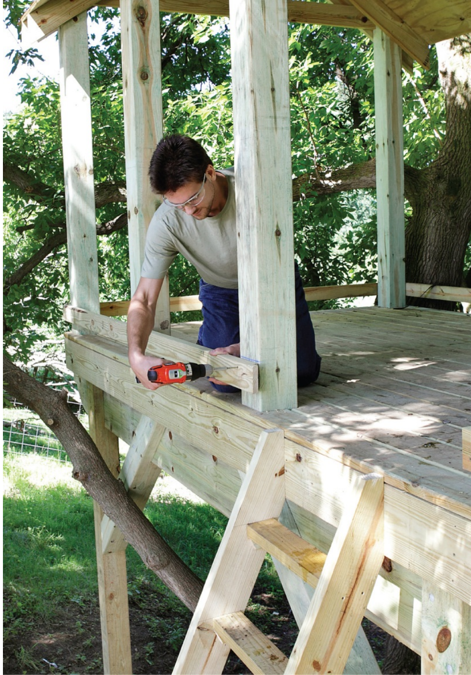
Install the rails with their top edges on the chalk lines. The 3" gap below the bottom rail makes it easy to sweep off the treehouse deck.
