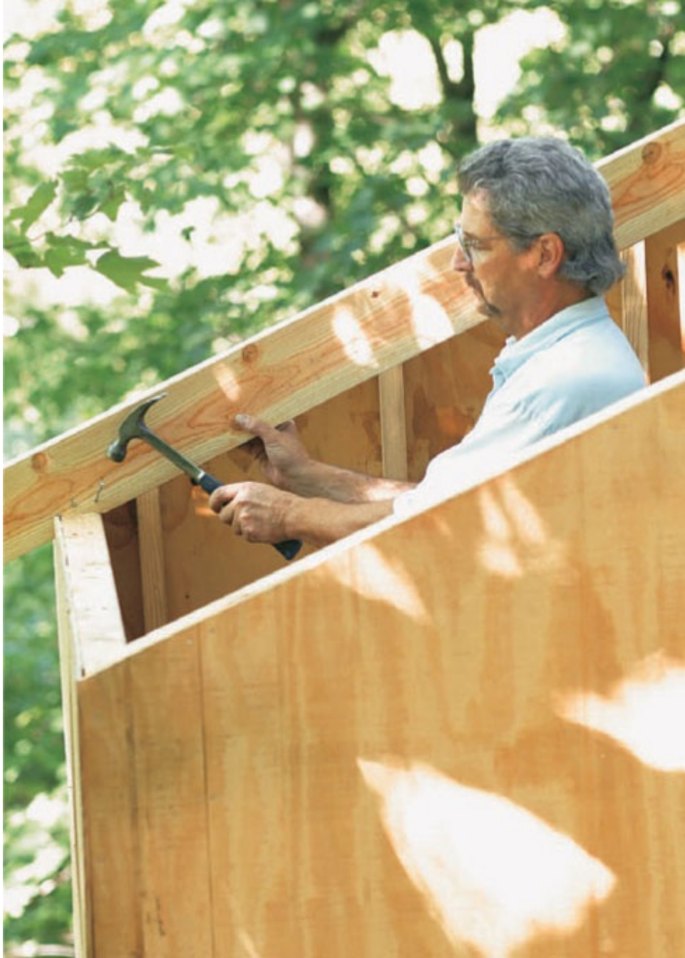
Toenail the rafters to the wall-top plates with three nails driven into the plates.
