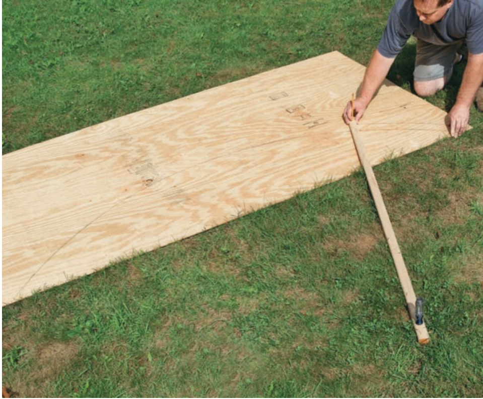
Use a trammel to mark the cutting lines for curved wall plates, pivoting the trammel from a centerline.
