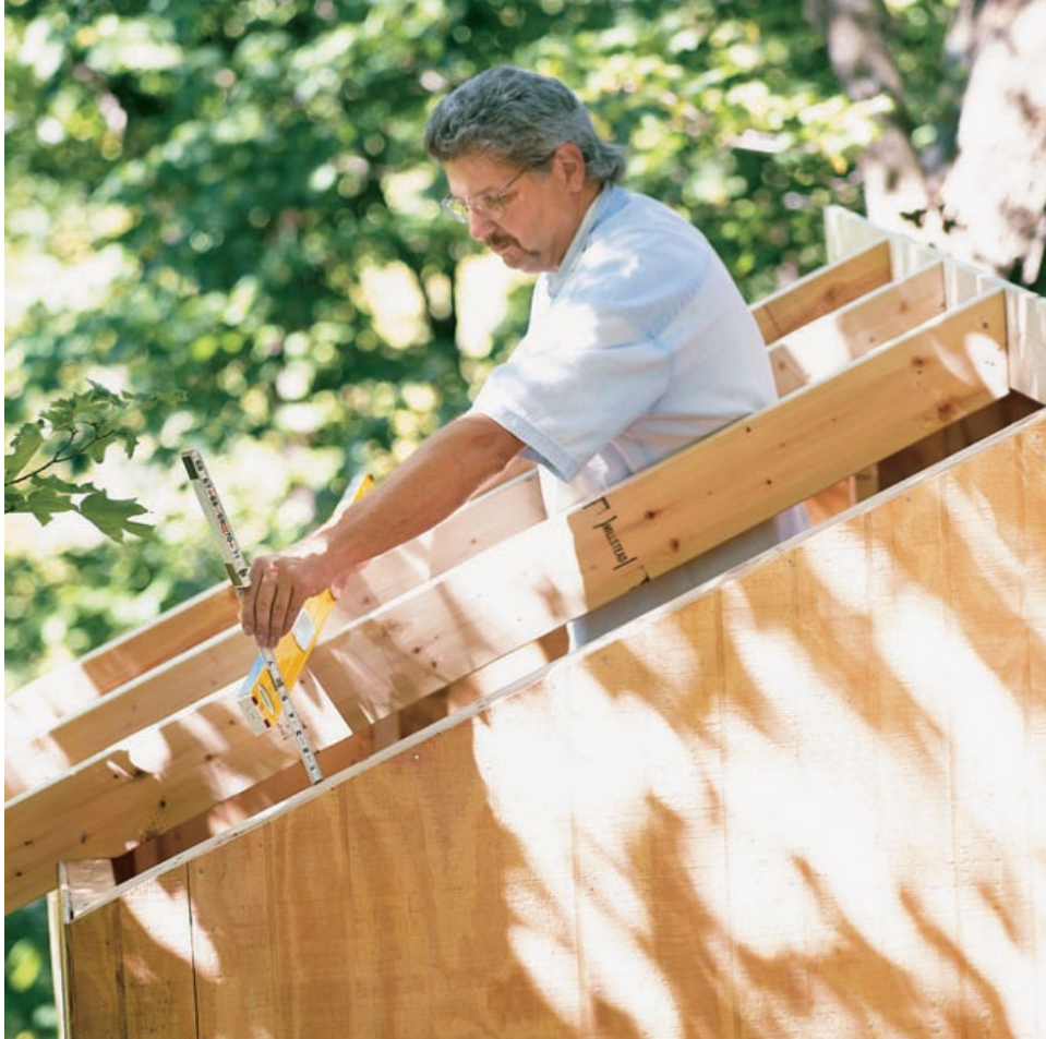
Level over from the inner rafters and measure to find the thickness of the outer rafters.
