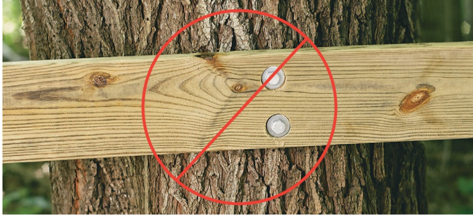
Fasteners placed close together in a vertical line can lead to rot in the tree, causing the anchors to fail.
