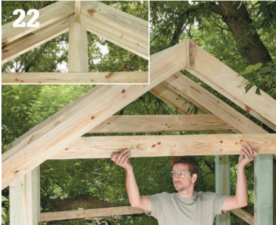
The gable-end rafter ties are combined with a strut to create a truss detail. The strut is notched to fit around the ridge beam (inset).
