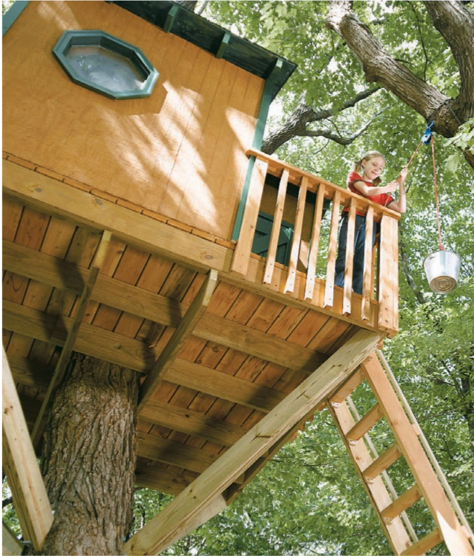
Self-closing hinges keep the gate shut when it's not in use—a handy safety feature for anyone using the treehouse.
