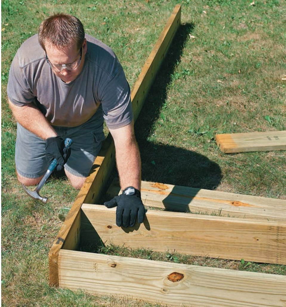
Build the 2 x 8 joist frame on the ground, then lift it up onto the platform beams.
