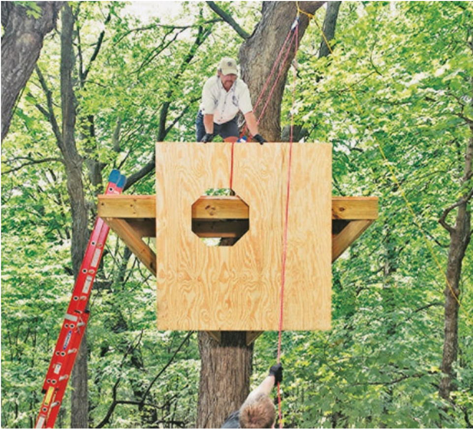
A block and tackle makes it easy to lift heavy support beams and pre-built walls.
