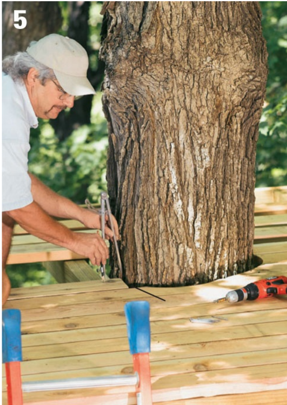
5 Custom fit the decking boards around the tree by butting each piece up to the tree and using a compass set at 2" to transfer the tree's contours to the board.
