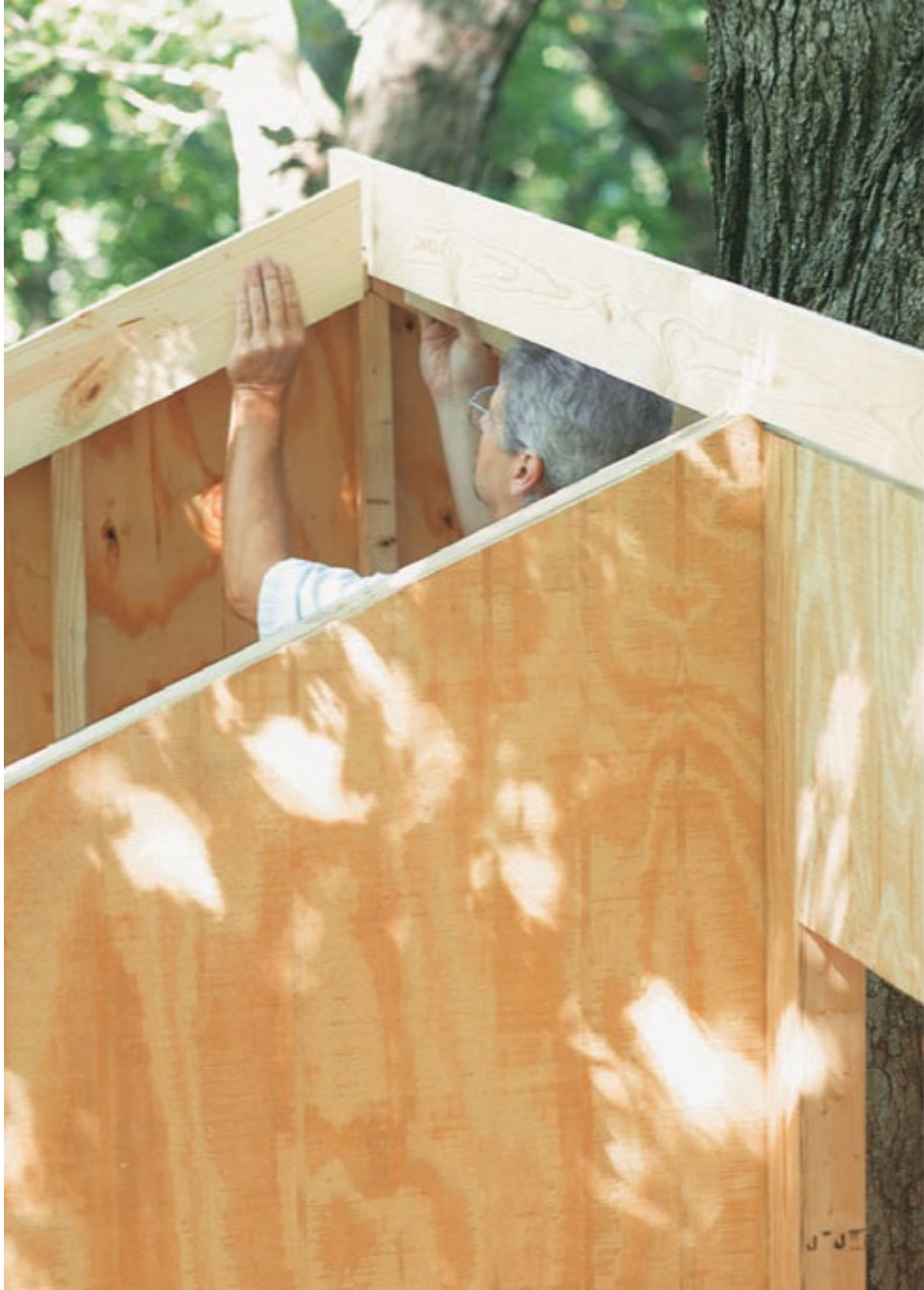
Test-fit the pattern rafters on the walls, using a scrap piece to act as the ridge beam.
