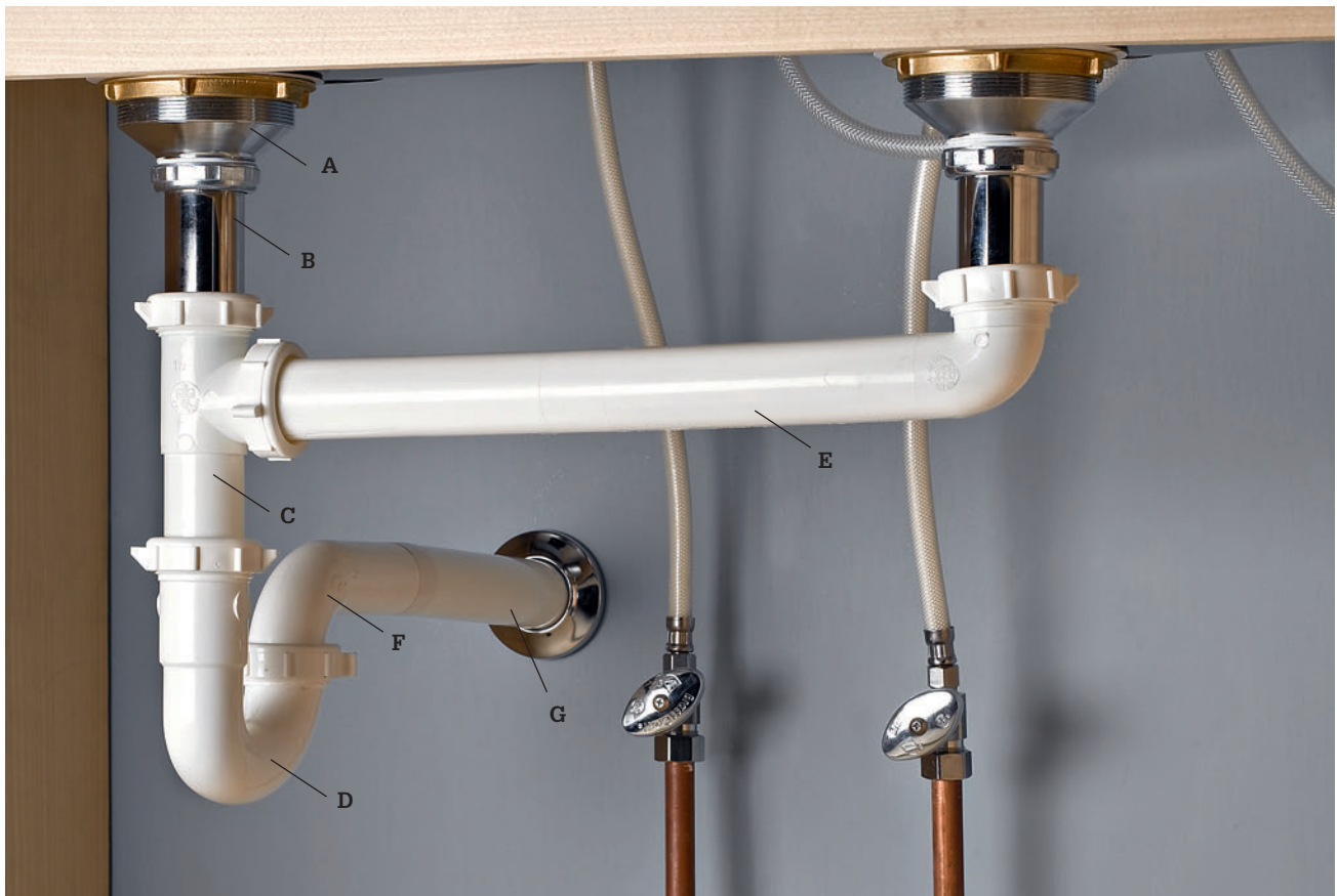
Kitchen sink drains include a strainer basket (A), tailpiece (B), continuous waste T (C), P- or S-trap (D), outlet drain lines (E), trap arm (F), and wall stubout (G).
