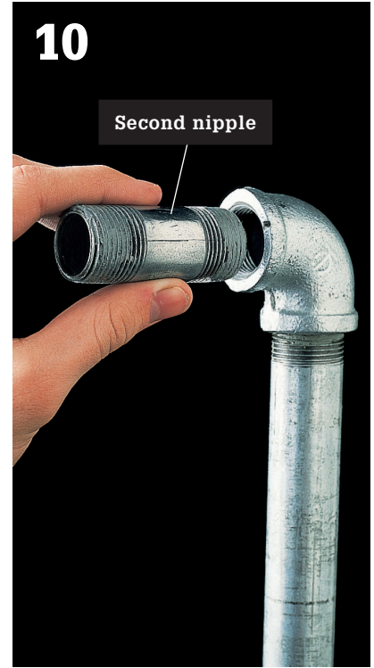
Screw the second nipple onto the other fitting. Tighten with a pipe wrench.
