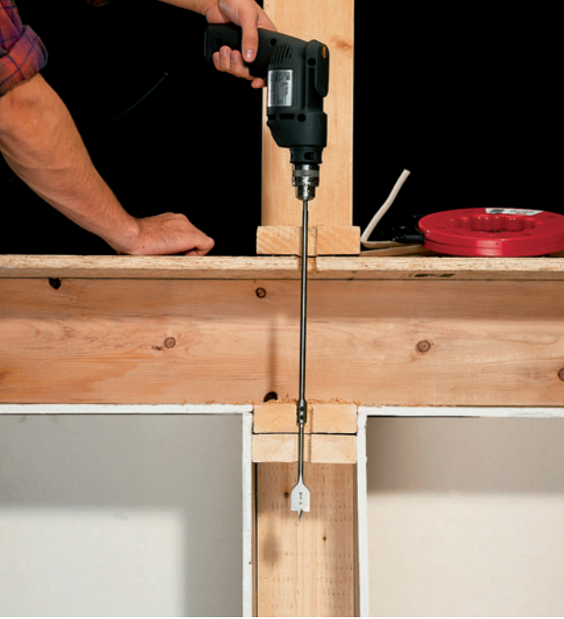
Use a drill bit extension and spade bit or hole saw to drill through wall plates from unfinished attic or basement spaces above or below the wall.
