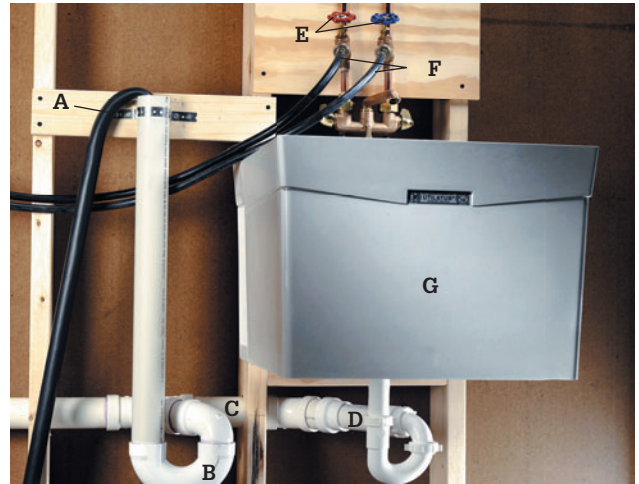
A washing machine with standpipe drain: washing machine drain hose (A), 2" standpipe drain with trap (B), waste line (C), utility sink drain pipe (D), hot and cold supply lines with hose bibs (E), rubber supply hoses to washing machine (F), and utility sink (G).
