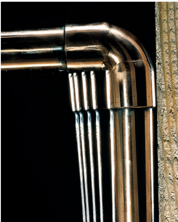
Clattering pipes can be a major annoyance, but they also should alert you of a problem with the supply system.
