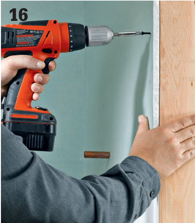
16 Install wallcovering material above the enclosure panels and anywhere else it is needed. Use moisture-resistant materials, and maintain a gap of ¼" between the shoulders of the top panel flanges and the wallcovering.
