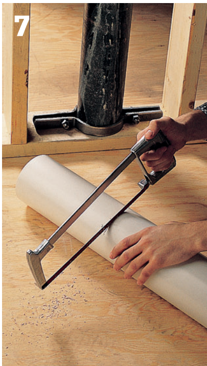
7 Cut a length of PVC plastic pipe to be ½" shorter than the section of cast-iron pipe that has been cut away.
