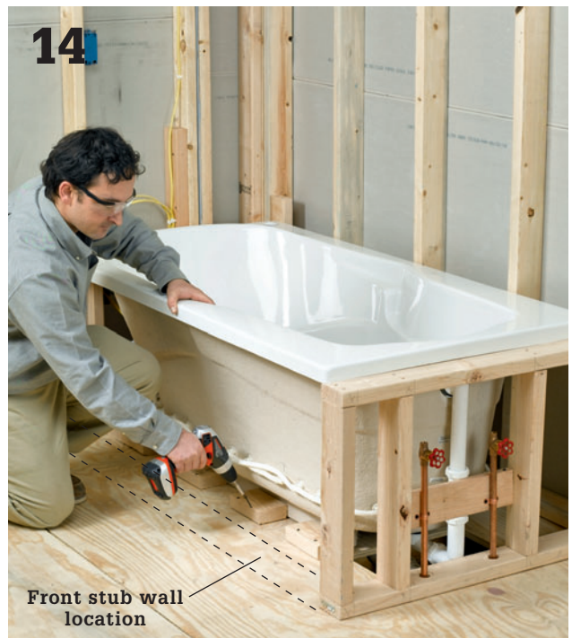
Secure the leveled tub in place as directed in your installation manual. Here, 2 × 4 block are screwed to the floor around the perimeter of the bathtub basin to create small curbs that prevent the tub from shifting. Build a 2 × 4 stub wall to support the front tub rim.
