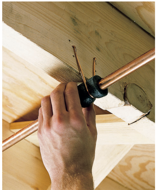
Loose pipes may bang or rub against joist hangers, creating noise. Use pieces of foam rubber pipe insulation to cushion pipes.
