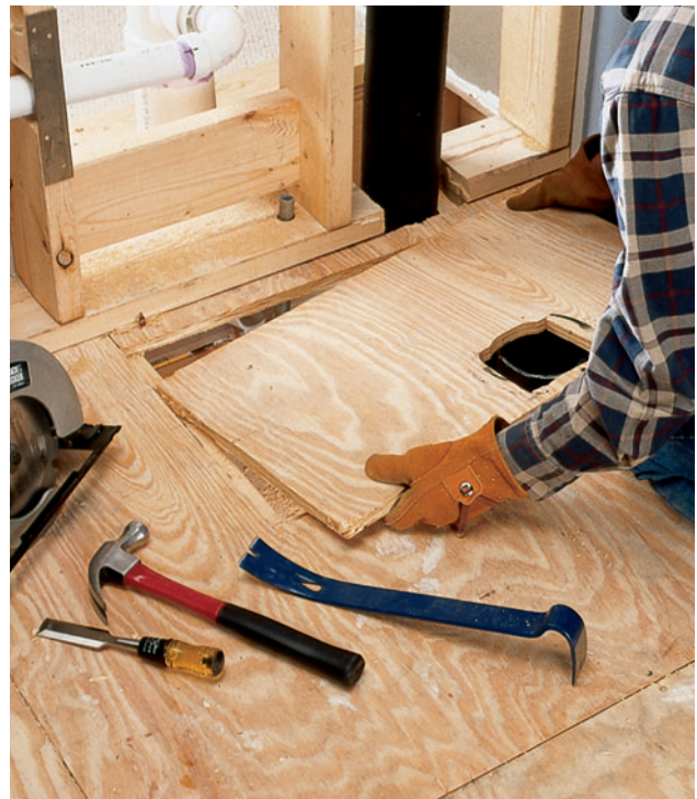
Replacing a toilet drain usually requires that you remove flooring and wall surface to gain access to the pipes.
