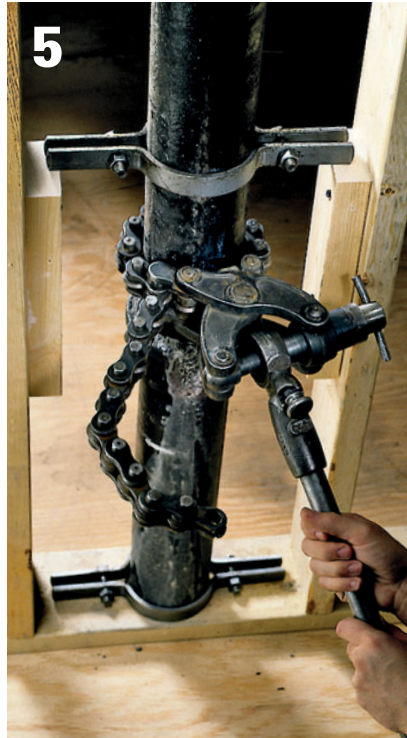
5 Tighten the chain and snap the pipe according to the tool manufacturer's directions.
