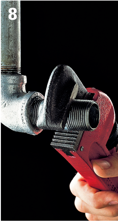
Screw the first nipple into the fitting, and tighten with a pipe wrench.
