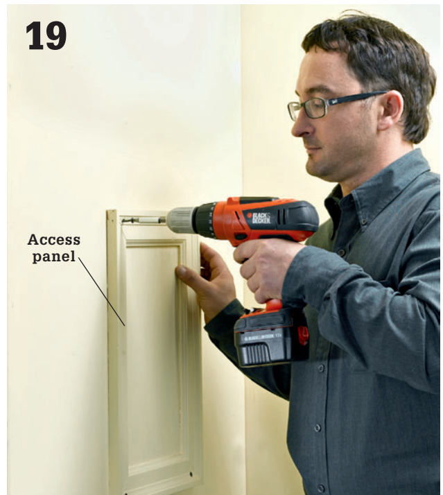
19 Make an access panel and attach it at the framed opening created in step 8. A piece of ¼" plywood framed with mitered case molding and painted to match the wall is one idea for access panel covers.
