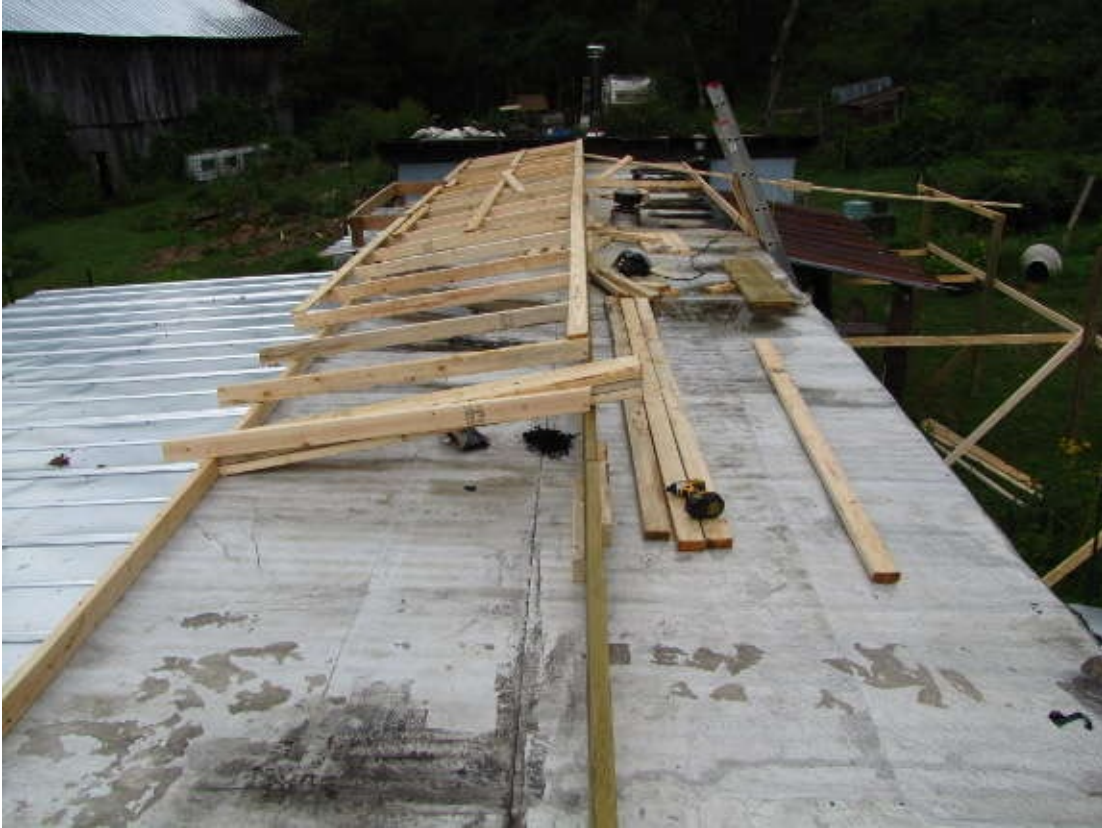
Propping the lower end of the rafters up on a two-by-four gave us room to include R30 insulation underneath most of the roof area.
