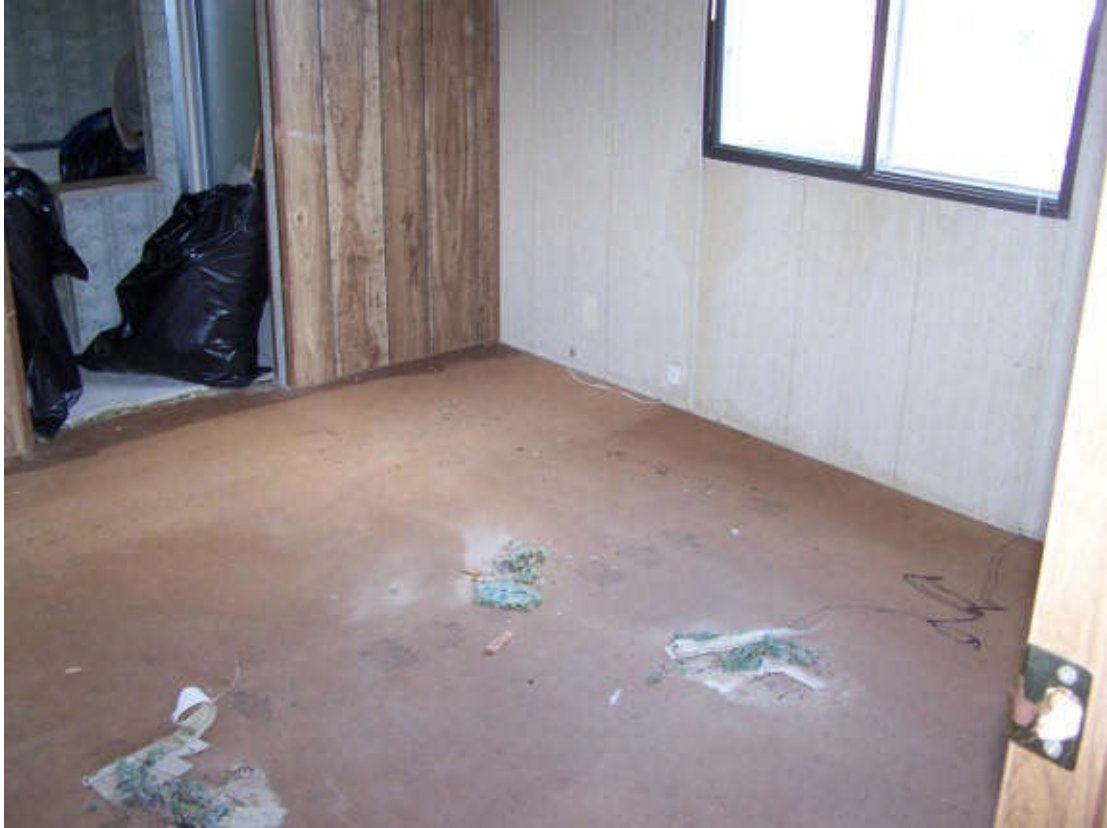
Jonathan and Andrea tore out the carpeting... Photo credit: Jonathan and Andrea Combs.
