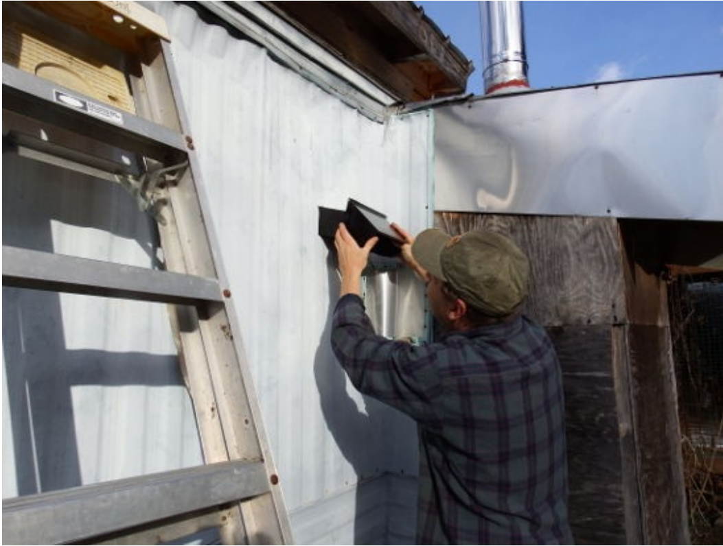
A duct wall cap goes through a hole in the exterior siding to attach directly into the back of the range hood.
