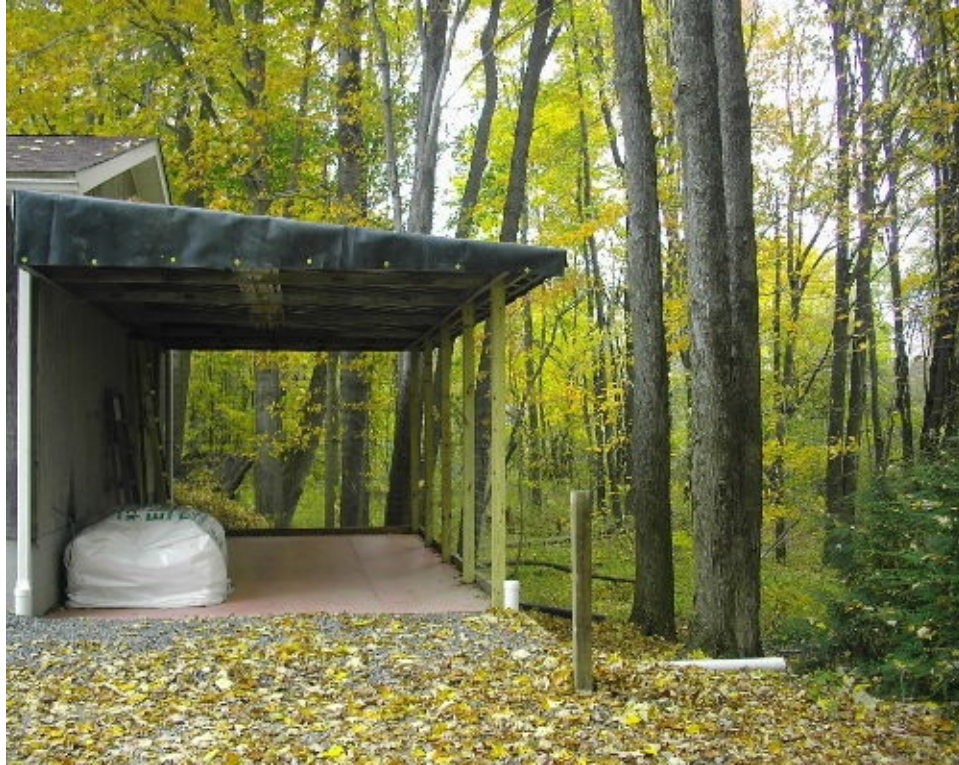
David and Mary built their new woodshed primarily using free materials. Photo credit: David and Mary.
