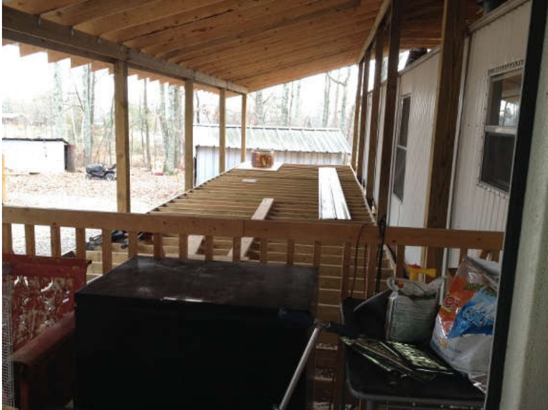
The roof allowed room for an extensive covered porch, which is still under construction. Photo credit: Lindsey and Keith.
