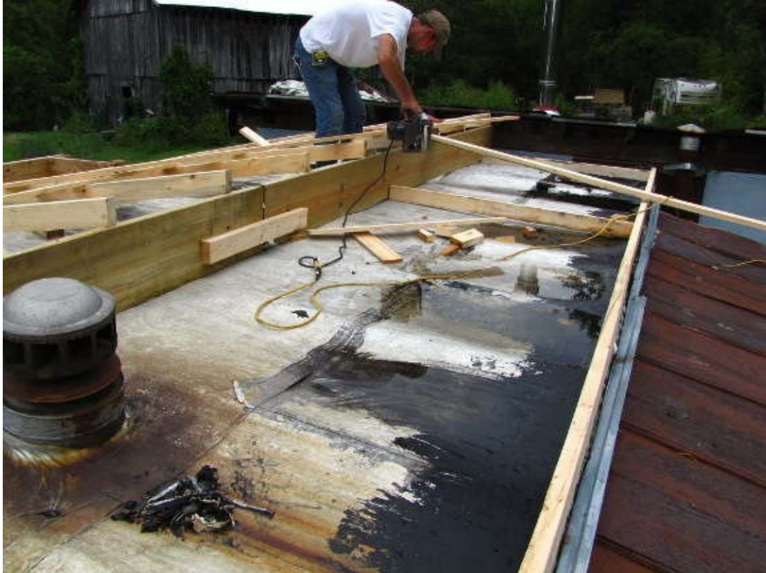
Our trailer started out with a nearly flat roof that allowed water to puddle on top of sagging tin.
