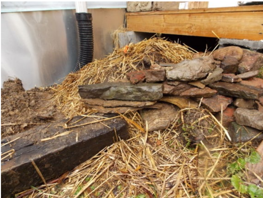
Water from some of our gutters flows into corrugated pipe that hooks into the
