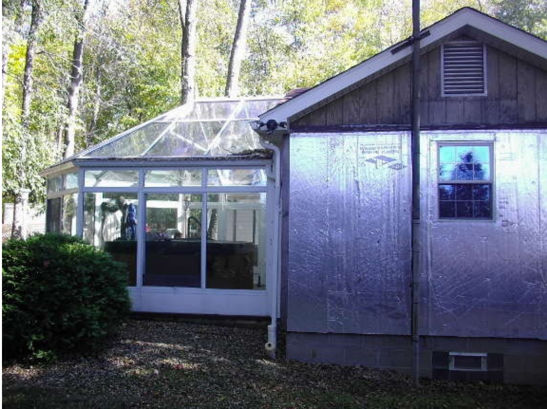
Adding rigid insulation to the outside of the wall is an easy way to increase thermal efficiency. Photo credit: David and Mary.
