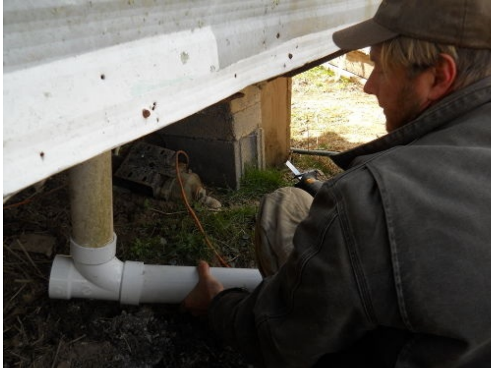
Our radical-plumbing job simply consisted of a pipe leading down from each sink basin, then a T sending the water downhill and into the wetland.
