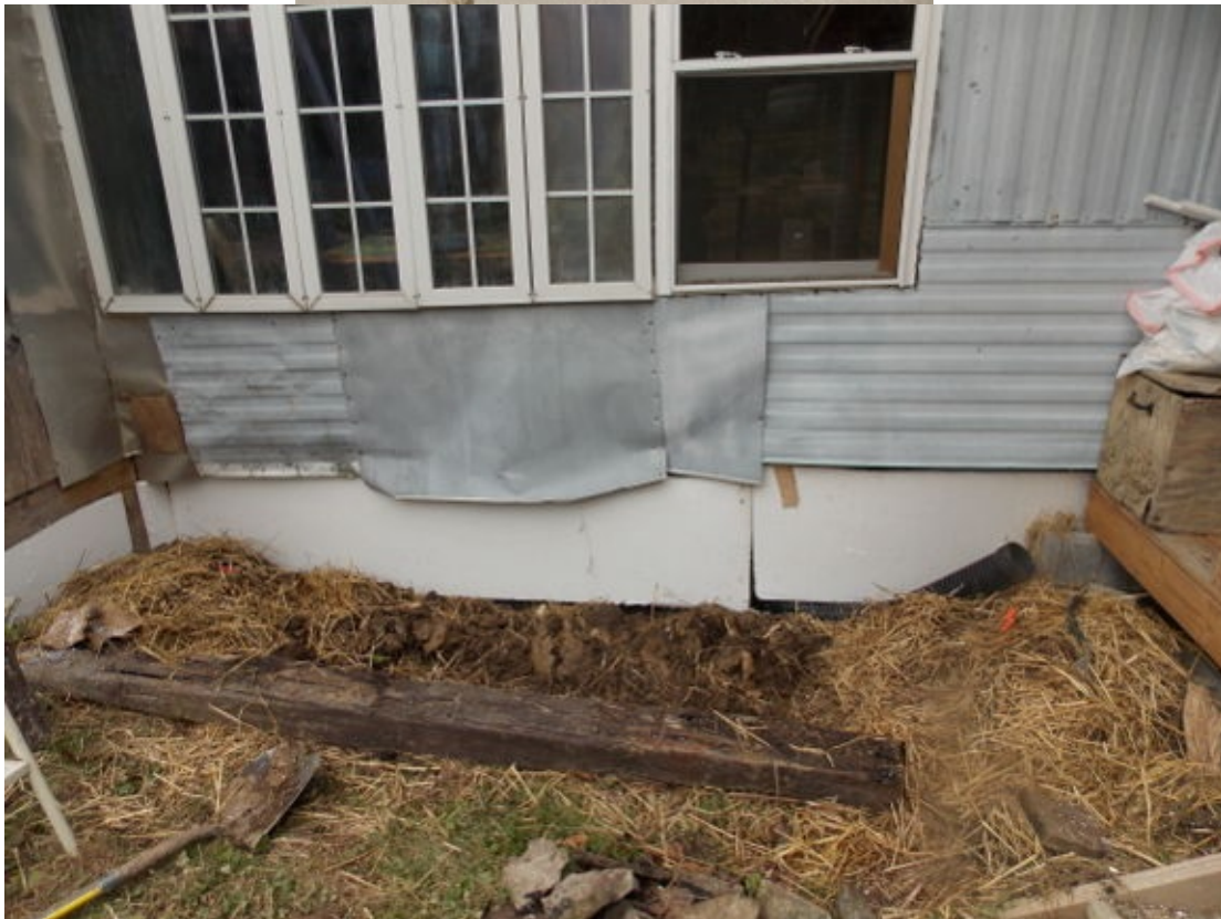
With the help of a scrap of wood, the insulation sheets slid into place without any special attachment.
