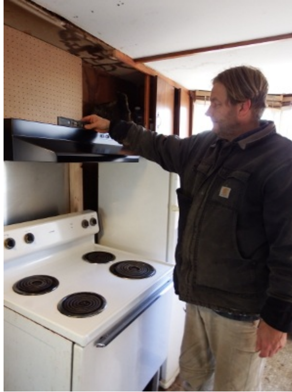
The finished stove hood is ready to suck pollutants out of the kitchen.
