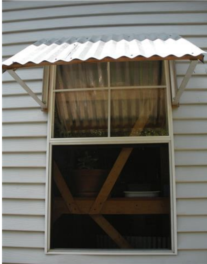
The awnings were constructed using metal roofing, aluminum angle, and treated wood. Photo credit: Harry and Zoe.
