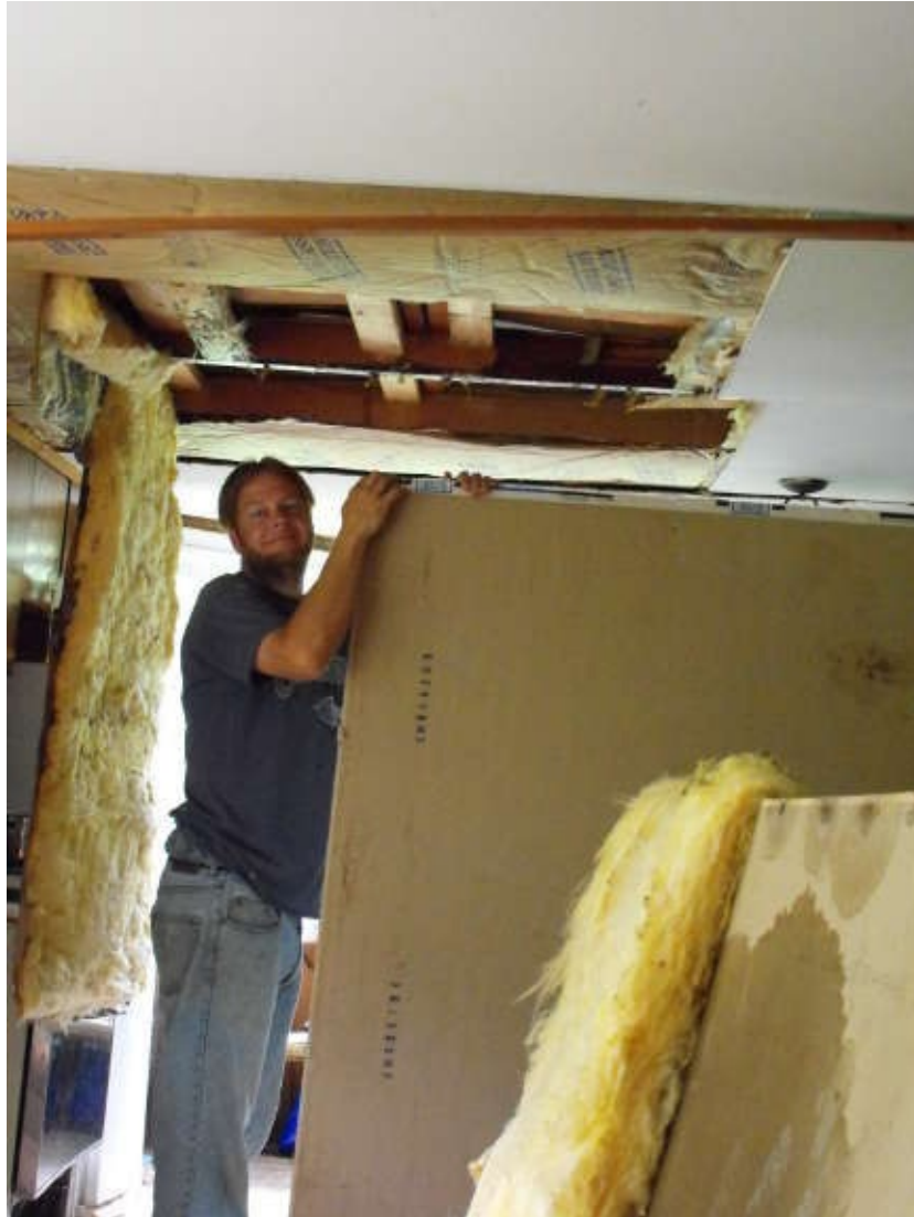
A leaky roof caused plenty of problems early in our trailer adventure. Here, Mark is replacing wet insulation after sealing a crack between sheets of roofing metal. Photo credit: Sara and Seth McDonald.
