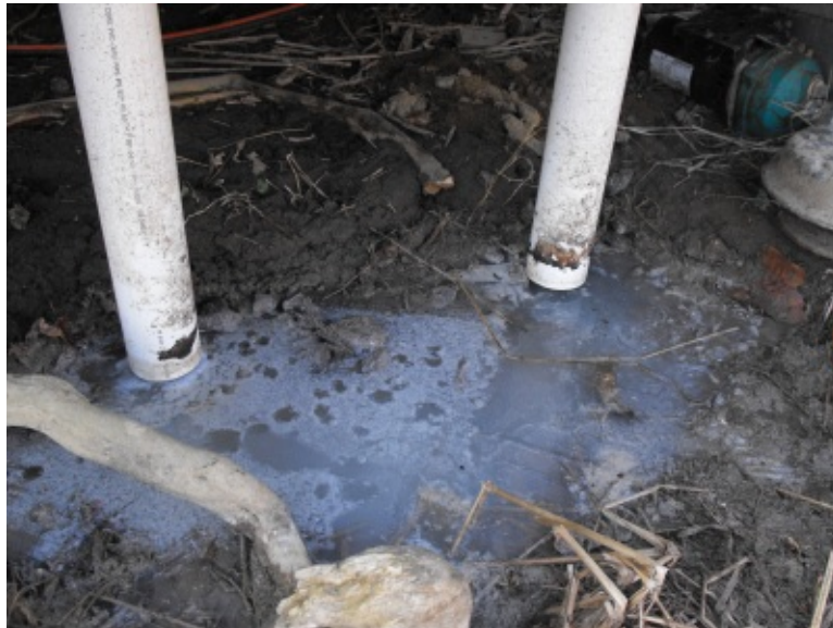
Our original drain out back was a muddy mess.
