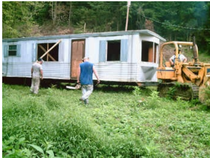
A bulldozer allows a trained crew to move trailers into the most surprising locations.
