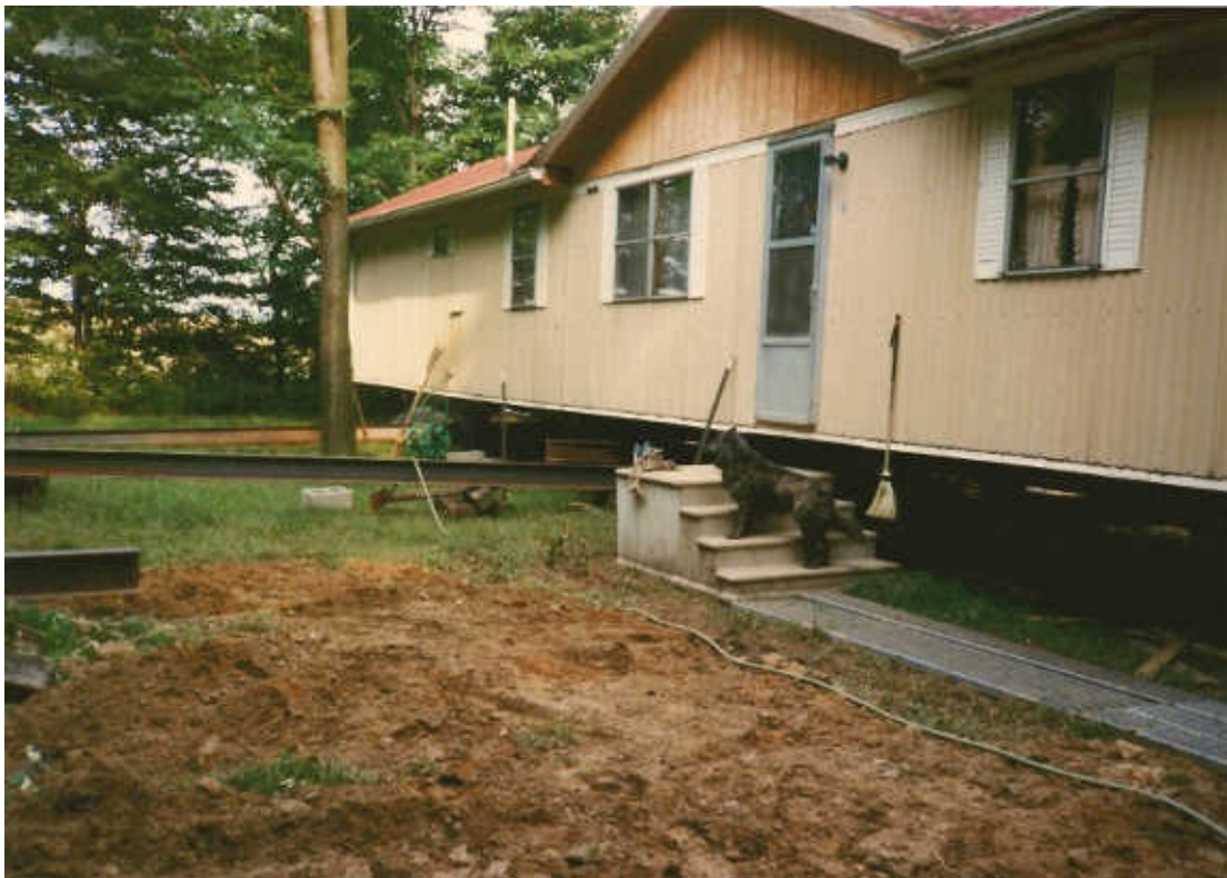
Their first major improvement was to contract out a pitched roof added onto
