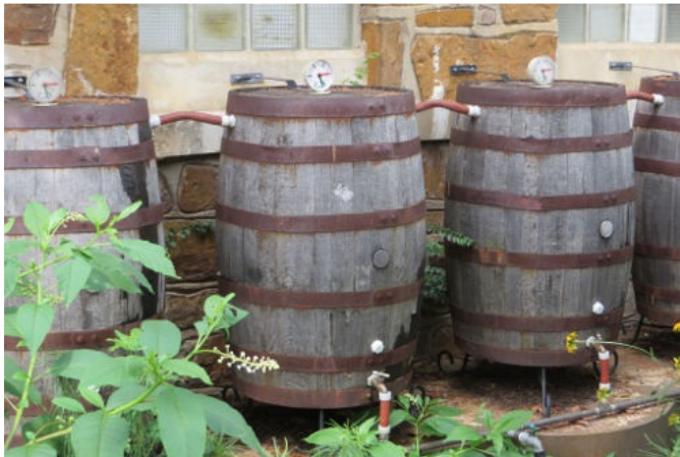
Daisy chaining multiple rain barrels together expands your water storage capacity. Photo credit: Brian Cooper, taken at the Little Rock Zoo.
