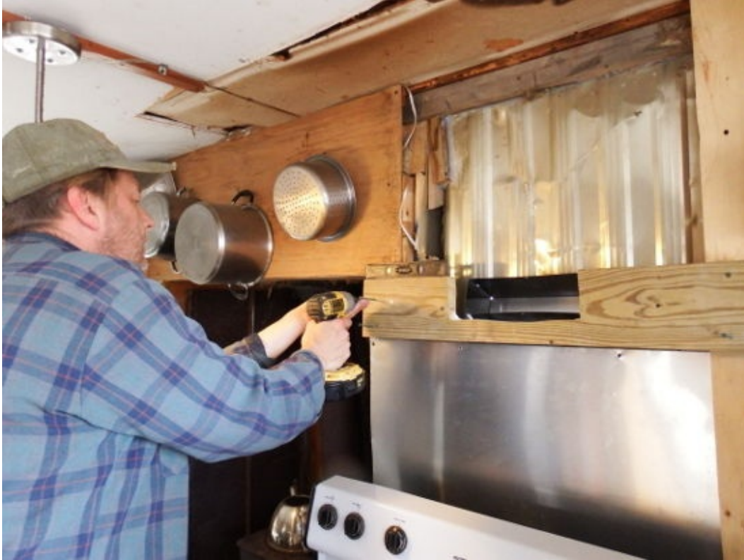
A two-by-six acts as a support for the range hood to screw onto.
