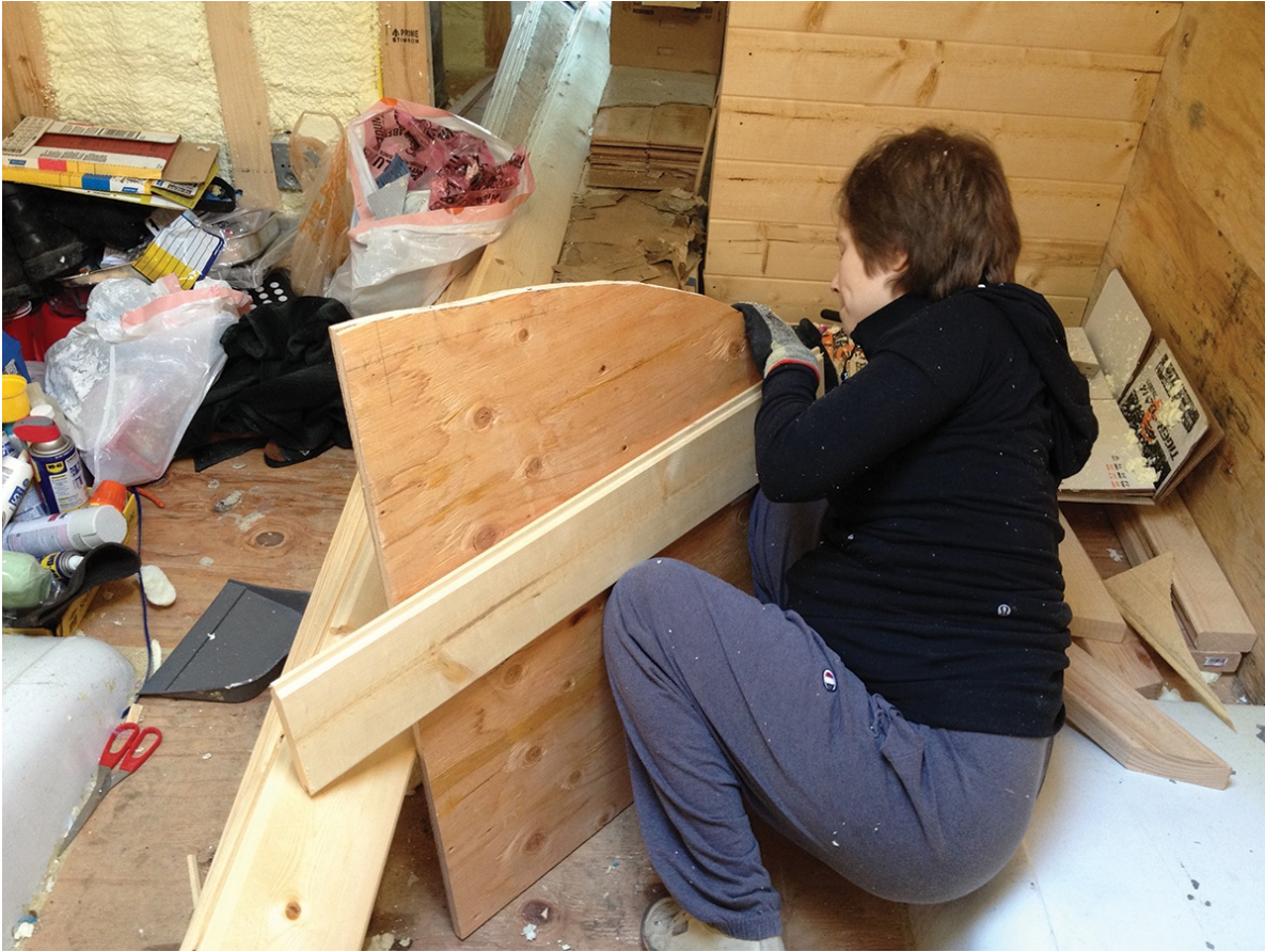
Starla Sullivan, using a contoured template of the roofline to mark out cuts in the wood paneling.
