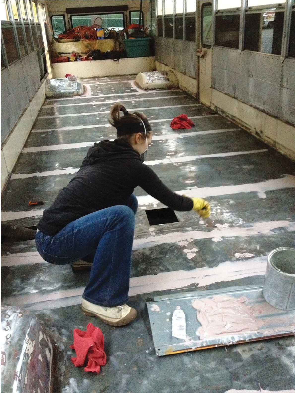
Removal of old flooring down to the metal, and preparation for a new coat of paint.
