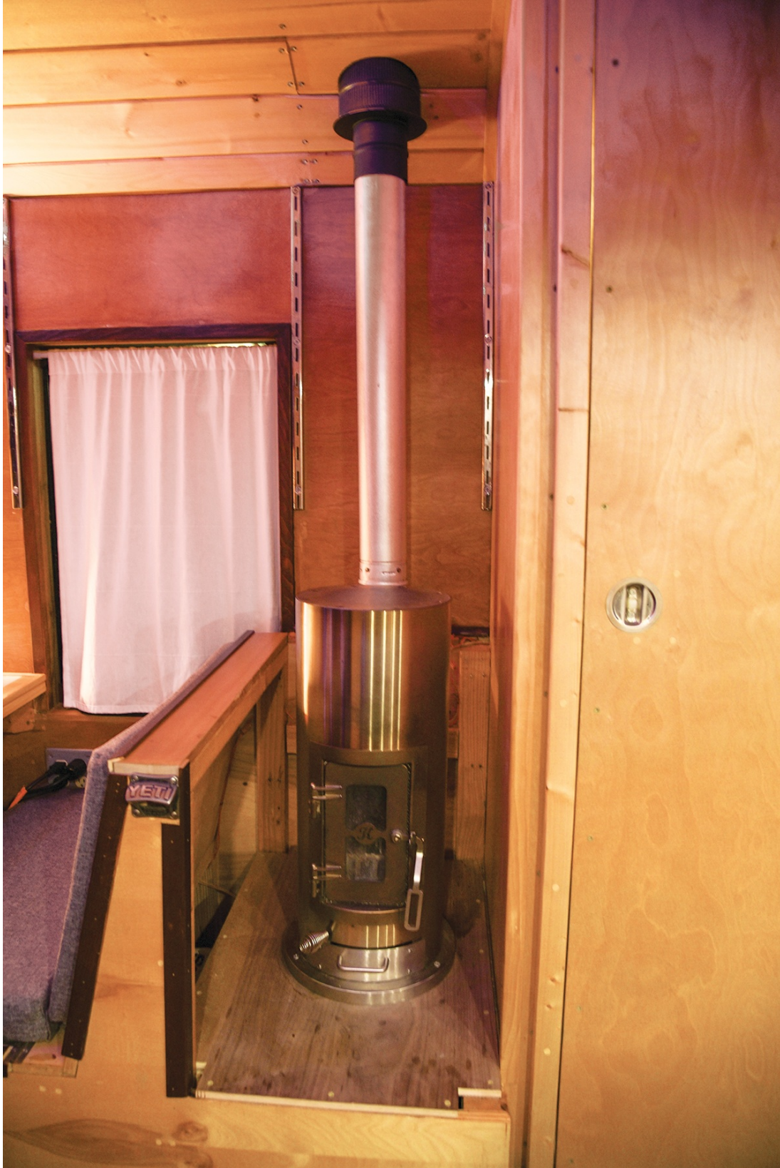
The bus uses a compact and ultra-efficient woodstove that's specially designed to fit into and heat up small spaces.
