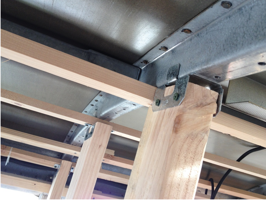
Using metal brackets to attach wood framing to the metal ribs of Big Bertha.
