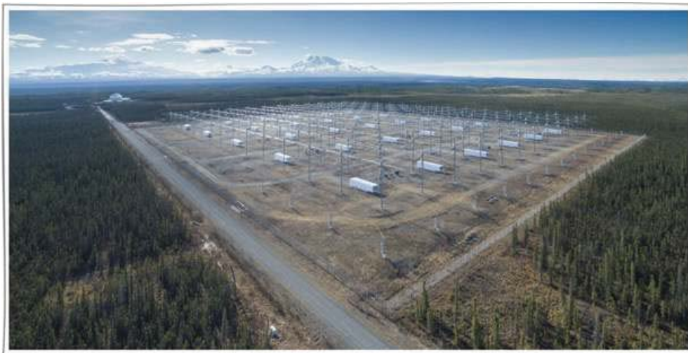
Antenna field for the HAARP system
