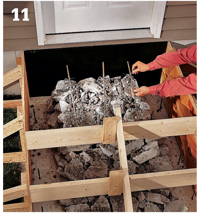
11 Lay pieces of #3 metal rebar on top of the fill at 12" intervals, and attach them to bolsters with wire to keep them from moving when the concrete is poured. Keep rebar at least 2" below the top of the forms. Mist the forms and the rubble with water.
