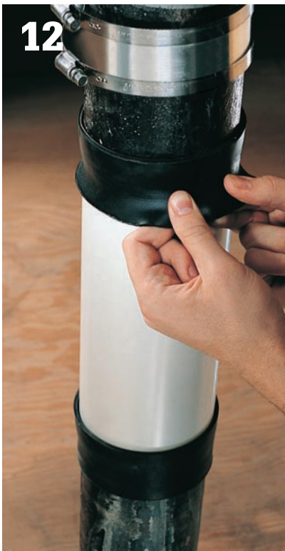
12 Roll the ends of the neoprene sleeves over the ends of the new plastic pipe.
