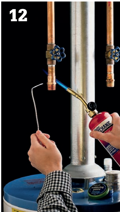
Solder threaded male adapters to the water pipes. Let pipes cool, then wrap Teflon tape around threads of adapters.
