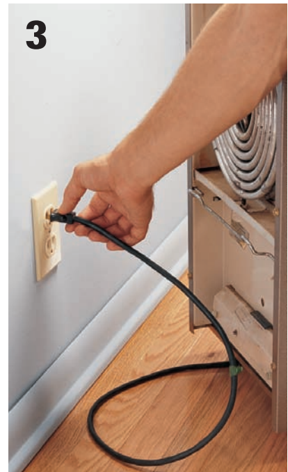
Disconnect all plug-in lamps and appliances from the receptacles.
