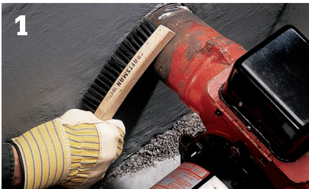
1 Use a wire brush to clean off any rust or dirt deposits that have accumulated on the surface.
