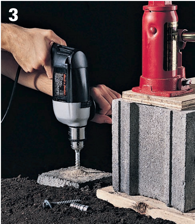
3 Drill a hole in the middle of the concrete pier, using a hammer drill and a \frac{5}{8} " masonry bit. Insert \frac{5}{8} " masonry anchor into hole.
