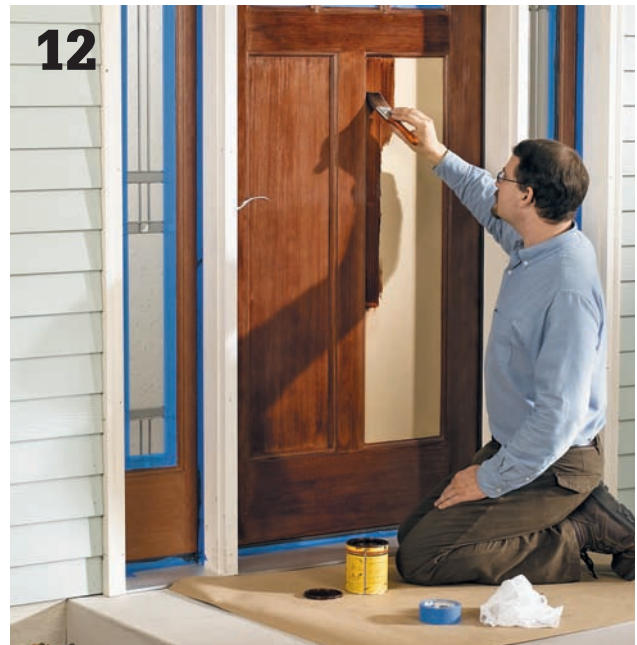
12 Apply your door finish if it has not yet been applied. Read the manufacturer's suggestions for finishing very closely and follow the suggested sequences. Some manufacturers offer finish kits that are designed to be perfectly compatible with their doors. Install interior case molding and caulk all the exterior gaps after the finish dries.
