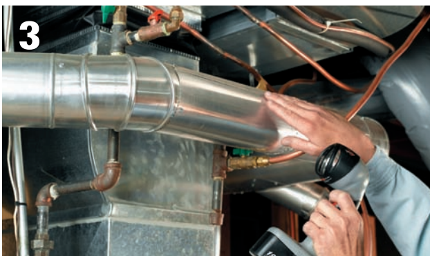
Inspect the areas around vent pipes for signs of corrosion. Corroded pipes will need to be replaced.
