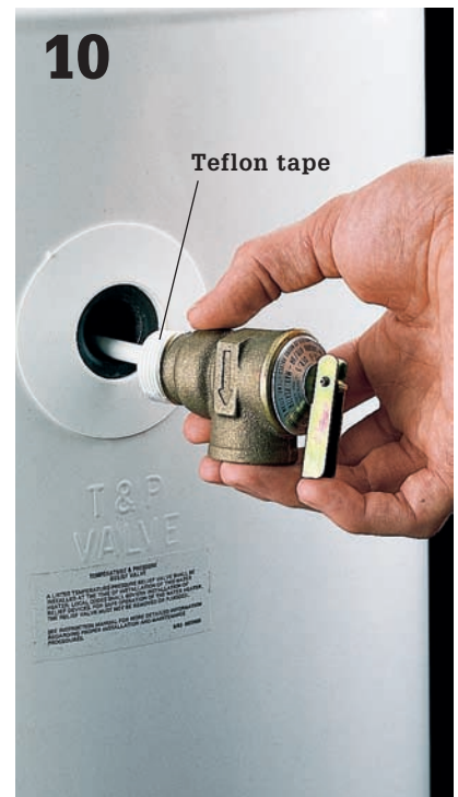
Wrap threads of new pressure-relief valve with Teflon tape, and screw valve into tank opening with a pipe wrench.
