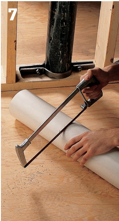
7 Cut a length of PVC plastic pipe to be 1/2" shorter than the section of cast iron pipe that has been cut away.
