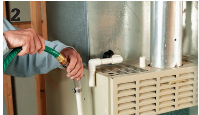
Clean the drain line once a year by running water through it from a garden hose.
