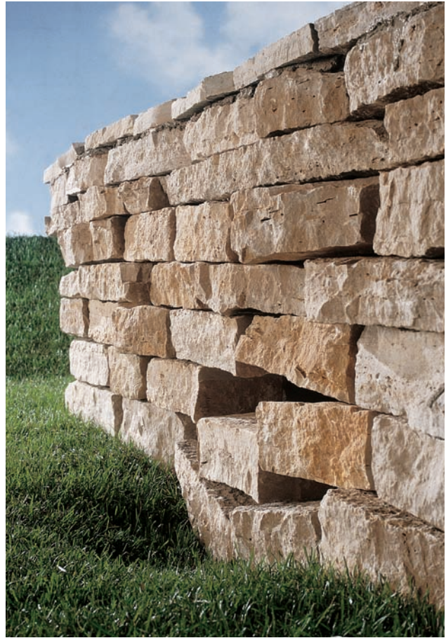
Stones in a wall can become dislodged due to soil settling, erosion, or seasonal freeze-thaw cycles. Make the necessary repairs before the problem migrates to other areas.
