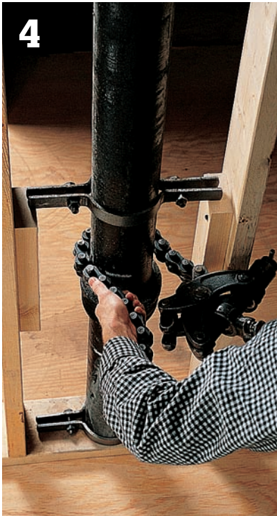
4 Wrap chain of the snap cutter around the pipe, so that the cutting wheels are against the chalk line.
