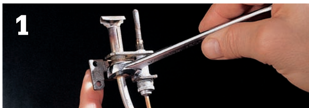
1 Loosen the connecting nut on the gas line with an open-end wrench.
