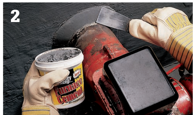
2 With a putty knife, apply refractory furnace cement to seal the leak.
