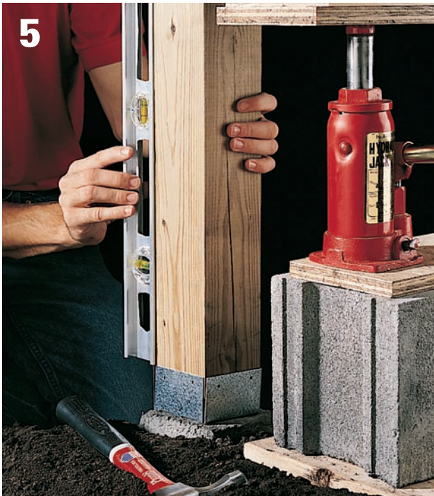
5 Cut new post from pressure-treated lumber, and treat cut ends with sealer-preservative. Position post and make sure it is plumb.
