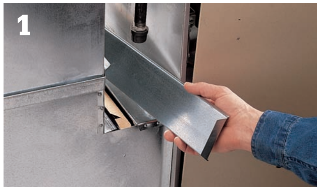
1 Many filters are located between the return air duct and the blower, and rest in a slot or bracket.
