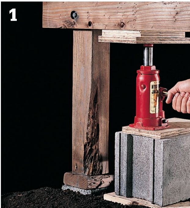
1 Build a support, using plywood scraps, a concrete block, and a hydraulic jack. Place 1½" layer of plywood between head of jack and beam. Apply just enough pressure to lift the beam slightly.
