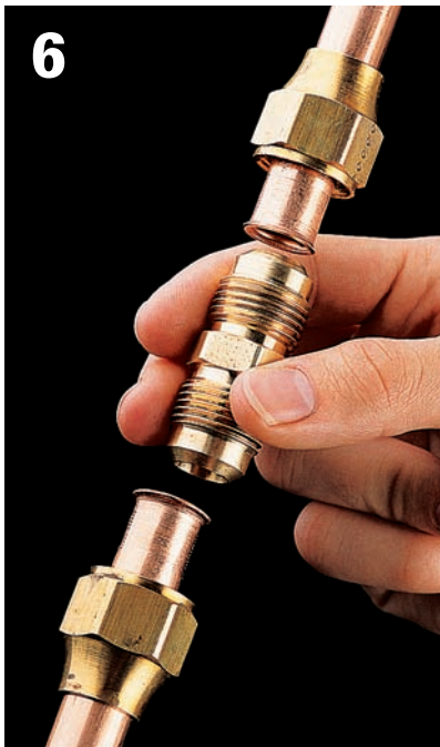
6 Place flare union between flared ends of pipe and screw flare nuts onto union.
