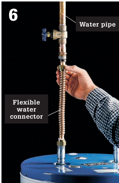
6 Connect water pipes and pressure-relief valve, following directions for gas water heaters (pages 395 to 396, steps 10 to 15). Open hot water faucets throughout the house, and turn on water. When water runs steadily, turn off faucets.
