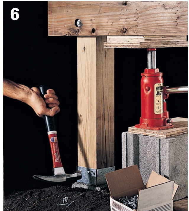
6 Attach the bottom of the post to the post anchor, using 10d or 16d joist hanger nails. Attach the post to the beam by redriving the lag screws, using a ratchet wrench. Release the pressure on the jack and remove the support.
