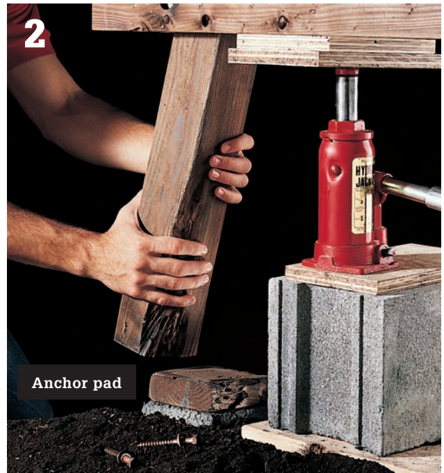
2 Remove the nails or lag screws holding the damaged post to the anchor pad and to the beam. Remove the damaged post and the wood anchor pad on the concrete pier.
