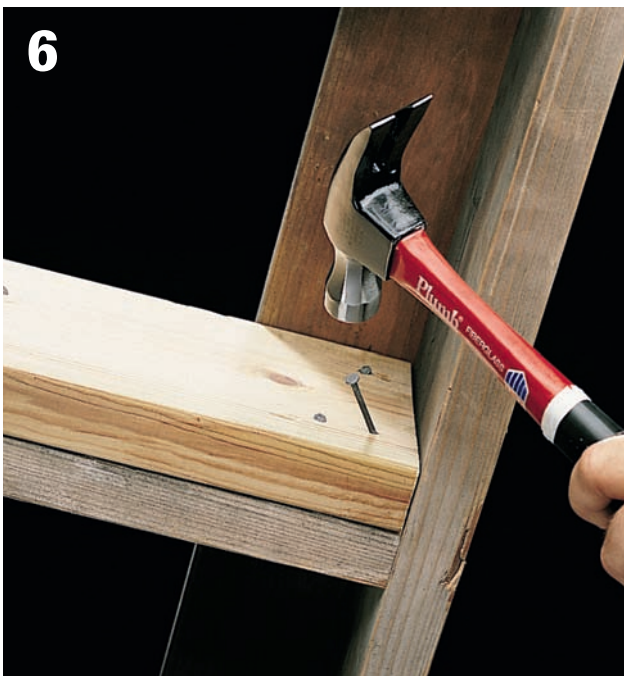
6 Attach sister joist to ledger and header joist by toenailing with 10d nails. Cut replacement decking boards from matching lumber, using a circular saw.
