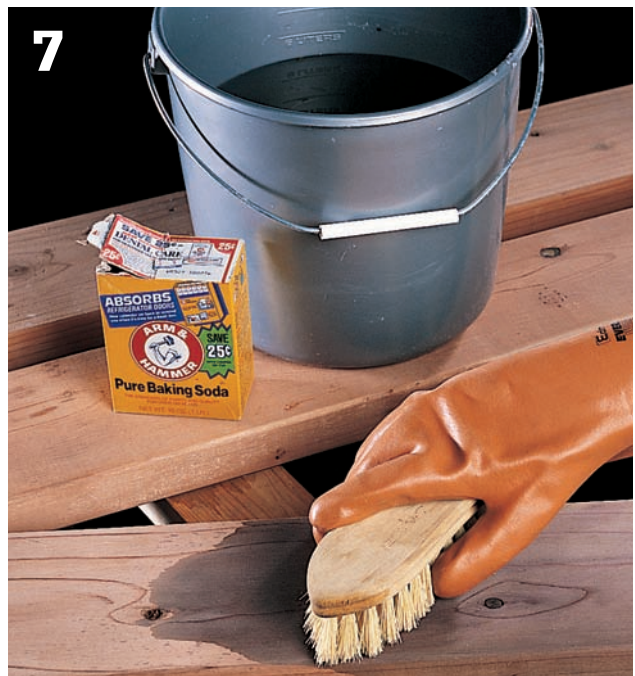
7 If the existing decking is gray, "weather" the new decking by scrubbing with a solution made from 1 cup baking soda and 1 gallon warm water. Rinse and let dry.
