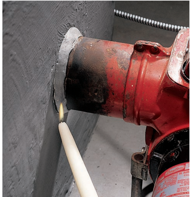
Hold a lighted candle to the joints on the flue and seams around the burner to find leaks.
