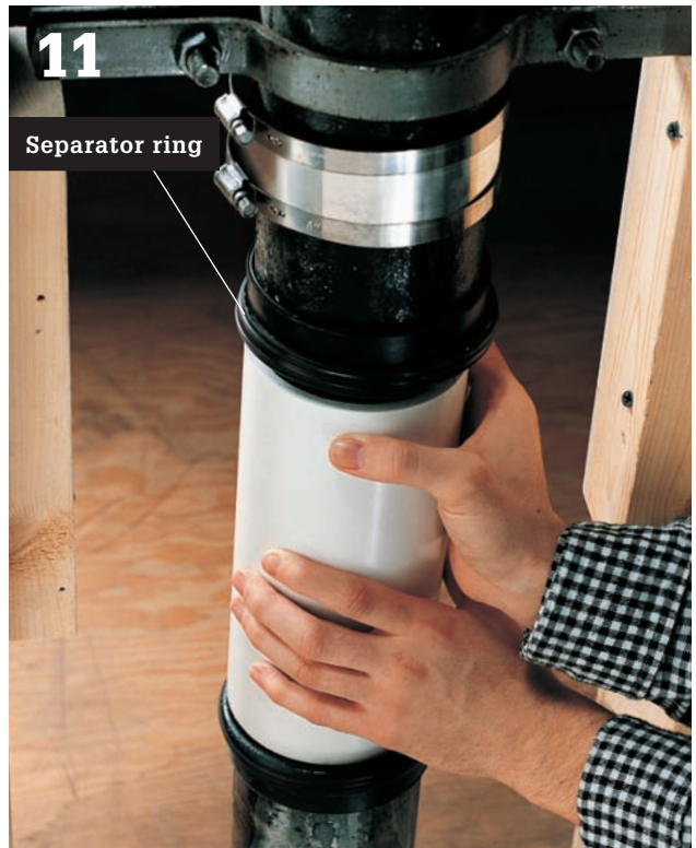
11 Position the new plastic pipe so it is aligned with the cast iron pipes.
