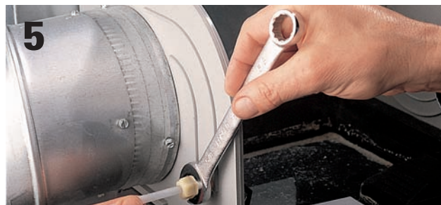
Adjust the float height and retighten the locknut.
