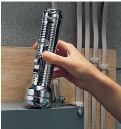
Keep a flashlight near your main service panel. Check flashlight batteries regularly.
