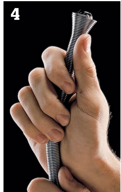
4 Bend chromed copper supply tube to reach from the tailpiece of the fixture to the shutoff valve, using a tubing bender. Bend the tube slowly to avoid kinking the metal.
