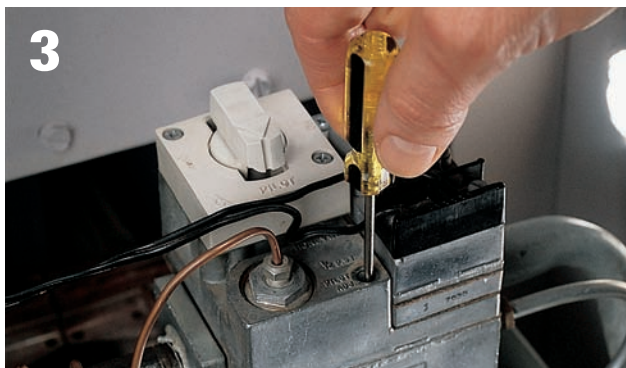
3 Turn the screw to adjust the height of the flame so it covers the top of the thermocouple.
