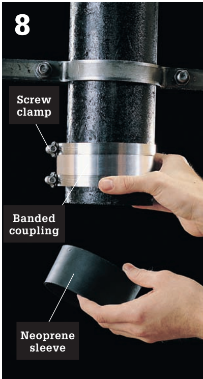
8 Slip a banded coupling and a neoprene sleeve onto each end of the cast iron pipe.
