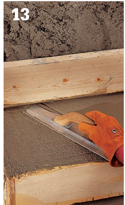
13 Float the steps , working the front edge of the float underneath the beveled edge at the bottom of each riser form.
