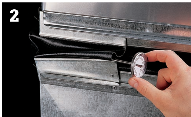
2 Check the temperature inside the supply duct and compare it with the temperature in the return duct.
