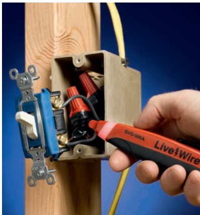
Always check for power at the fixture you are servicing before you begin any work.
