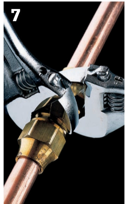
7 Hold center of flare union with adjustable wrench and use another wrench to tighten flare nuts one complete turn. Turn on water. If fitting leaks, tighten nuts.
