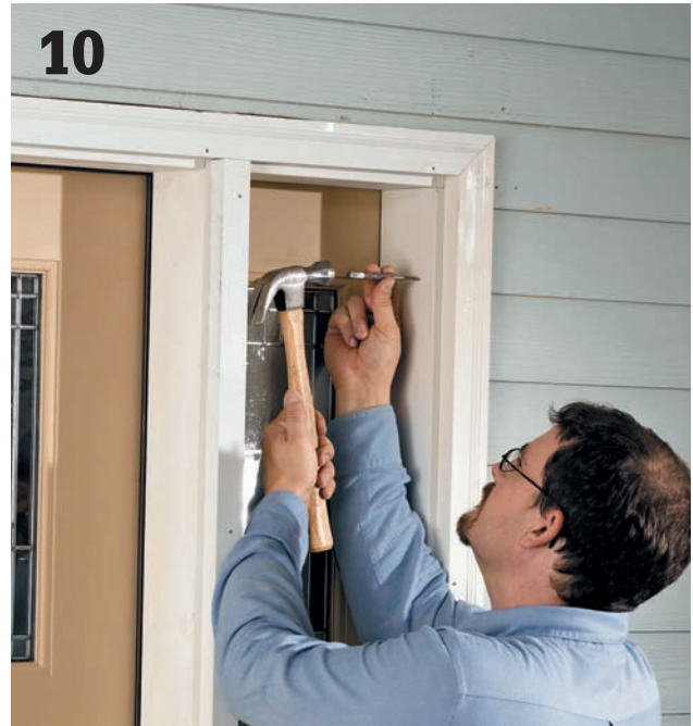
10 Use a nail set to drive the nail heads below the wood surface. Fill the nail holes with wood putty (you'll get the best match if you apply putty that's tinted to match the stained wood after the finish is applied). The presence of the wood shims at the nail locations should prevent the jamb from bowing as you nail.
