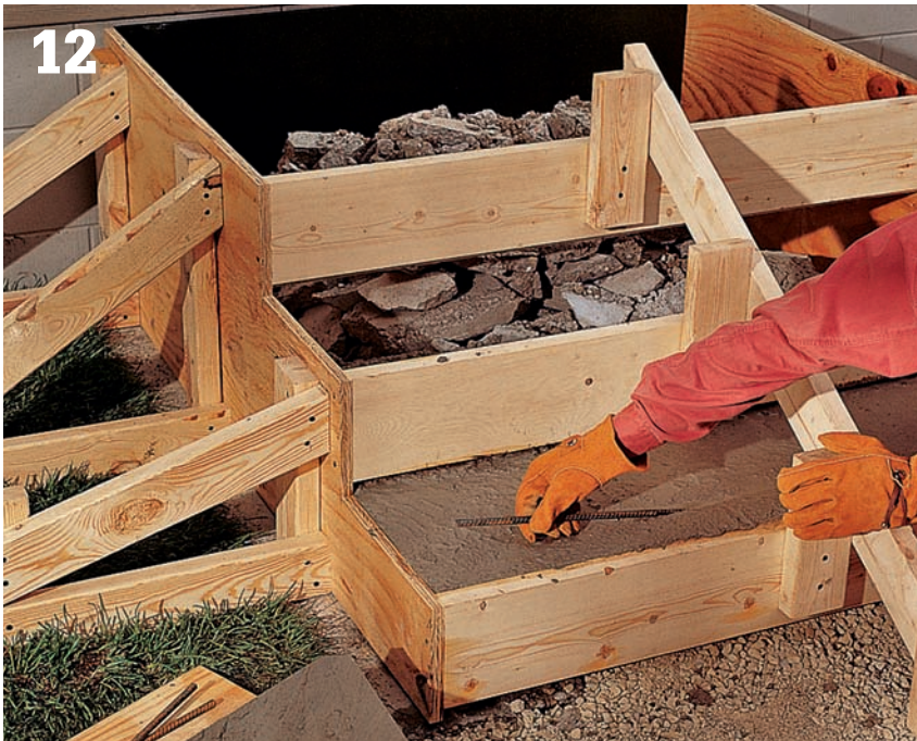
12 Coat the forms with vegetable oil or a commercial release agent , then mist them with water so concrete won't stick to the forms. Mix concrete and pour steps one at a time, beginning at the bottom. Settle and smooth the concrete with a screed board. Press a piece of #3 rebar 1" down into the "nose" of each tread for reinforcement.
