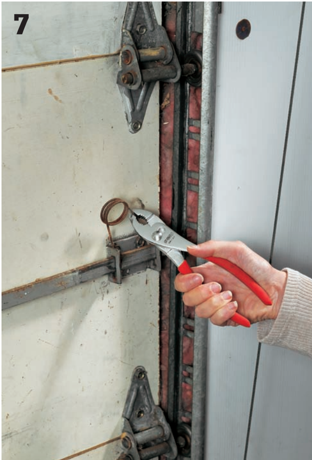
7 Sometimes the door lock bar opens sluggishly because the return spring has lost its tension. The only way to fix this is to replace the spring. One end is attached to the body of the lock; the other end hooks onto the lock bar.
