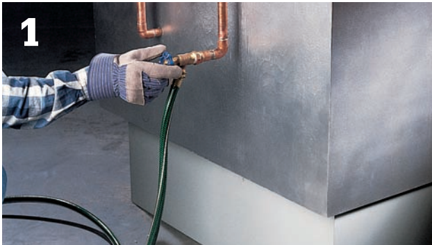
1 Use a garden hose to drain water from the boiler. Keep the drain end of the hose lower than the drain cock on the boiler.
