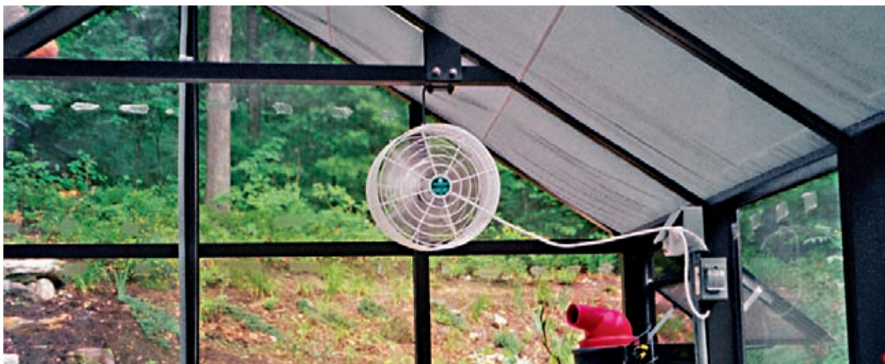
Roof shades , along with vents, help prevent a greenhouse from overheating in direct sunlight. Here, a combination of circulating fans and cloth shades mounted on the interior of the south-facing glass helps protect plants.
