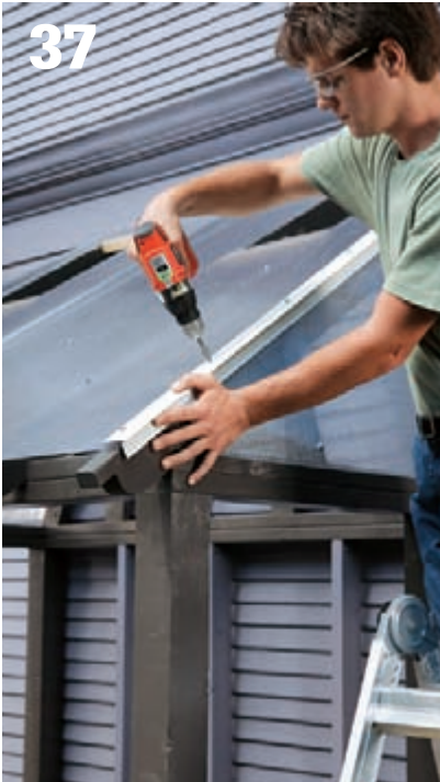
37 Install flashing over the hip roof seams. Here, common drip cap flashing is being fastened with rubber-gasket screws driven into the roof rafters.
