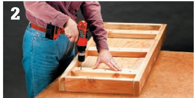
2 Position the frame over the subbase and fasten it by driving 2" deck screws through the stretchers and into the plywood. Also drive some screws down through the cementboard underlayment and plywood and into the stretchers.
