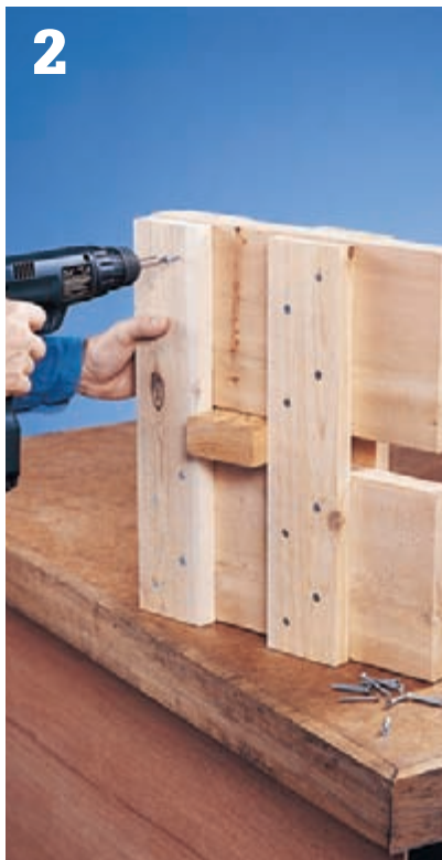
2 Attach the remaining leg half to the cleats on both ends, sandwiching the trestle on all sides.
