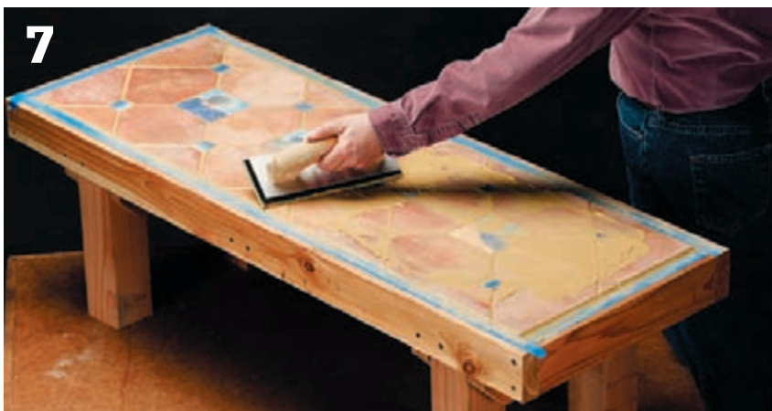
Mix a batch of grout and use a grout float to force it into the joints between tiles. Buff off the excess once the grout sets up.
