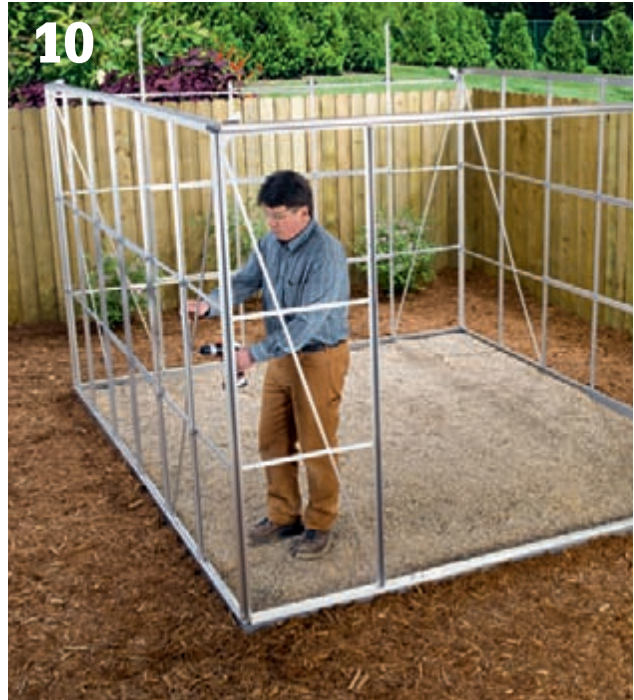
10 Add diagonal struts , as directed by the manufacturer. The struts help to stiffen and square up the walls. As you work, take diagonal measurements between opposing corners at the tops of the walls, to make sure the structure remains square.
