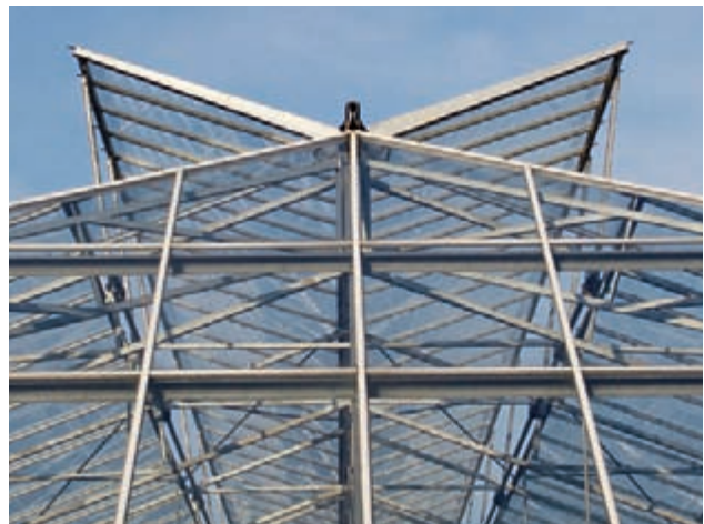
Roof vents that are triggered to open automatically by sensor alerts are far and away the most important component of a greenhouse cooling system. But additional cooling devices may be necessary.
