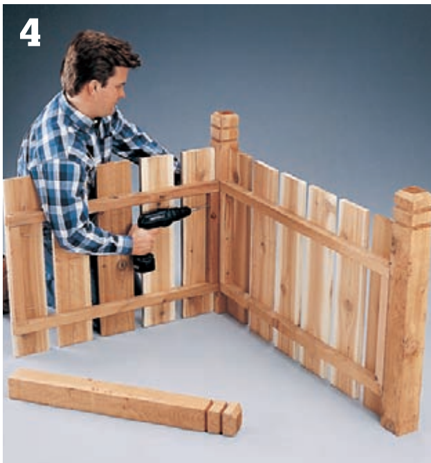
Stand the posts and panels upright, and fasten the panels to the posts by driving screws through the cleats.
