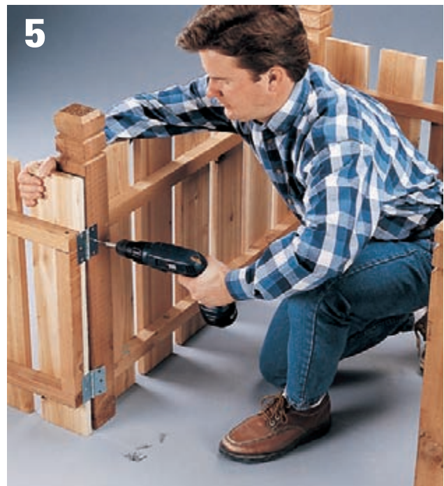
Attach exterior-rated hinges to the end panel frame and then fasten them to the post. Add a latch on the other side of the hinged panel.
