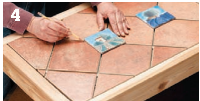
4 Dry-fit the field tiles using tile spacers to set consistent gaps. Set the accent tiles in place and mark the field tiles for cutting.
