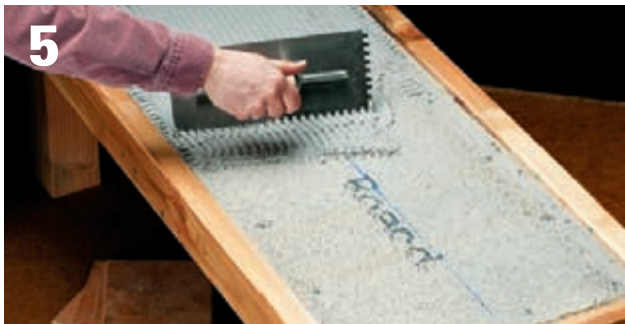
Apply a setting bed of thinset mortar onto the cementboard using a notched trowel.
