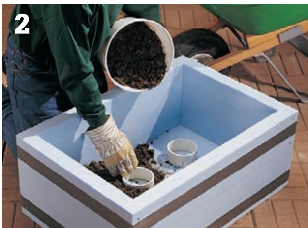
Pack hypertufa onto the floor of the form; press it down firmly to create a level, 2"-thick floor.
