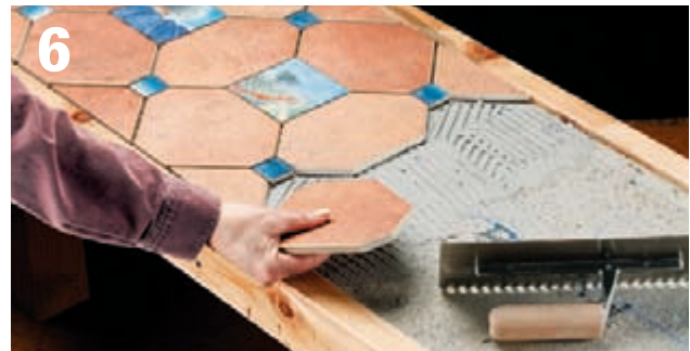
Set the tiles into the thinset mortar using a slight twisting motion as you press down.
