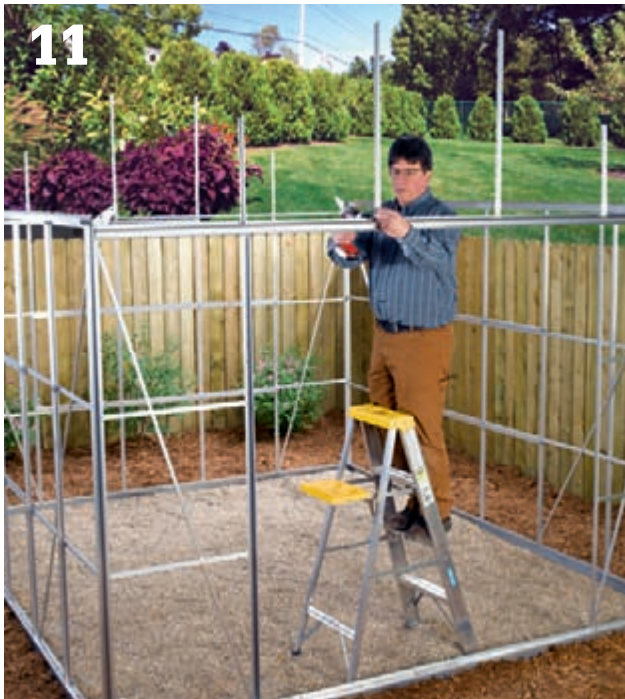
11 Fasten the gable-end stud extensions to the front and back walls of the greenhouse. The top ends of the studs should angle upward, toward the peak of the greenhouse.
