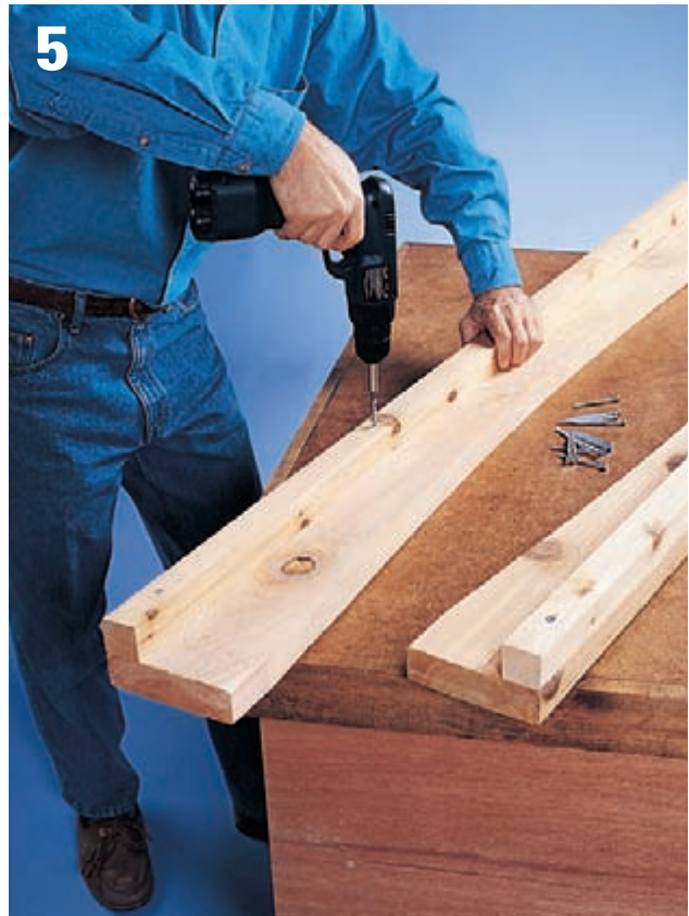
5 Attach a 2 x 2 slat to the top inside edge of each apron using 2½" deck screws and glue.
