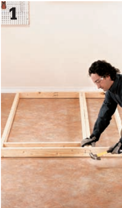
1 Build the wall frames. For the front wall, attach the plates to the outside studs first and then attach the inside studs using the door header as a spacer to position the inside studs.
