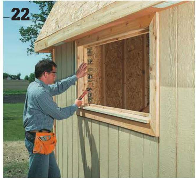
22 Build the window frame, which should be \frac{1}{2} " narrower and shorter than the rough opening. Install the frame using shims and 10d galvanized casing nails, as shown in the WINDOW JAMB DETAIL (page 146). Cut eight 1 x 2 stop pieces to fit the frame. Bevel the outer sill stop for drainage. Order glass to fit, or cut your own plastic panel. Install the glazing and stops, using glazing tape for a watertight seal. Add the window trim.
