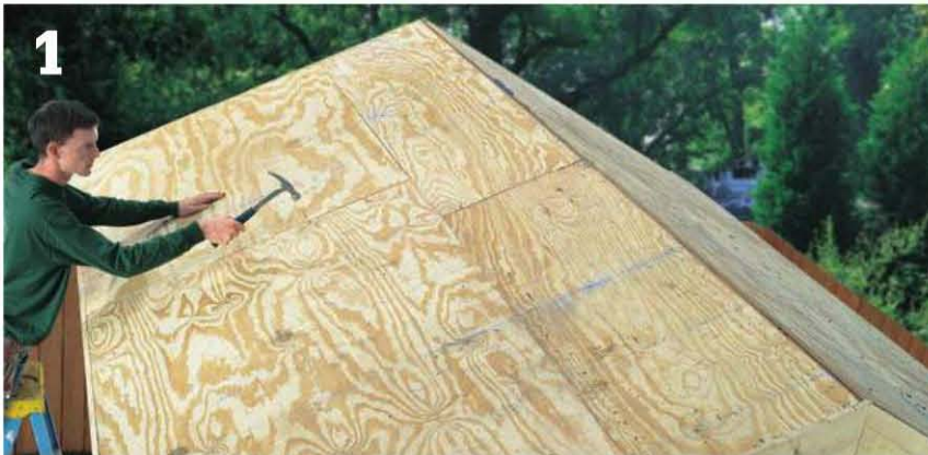
Install the plywood sheathing so the vertical joints are staggered between rows.
