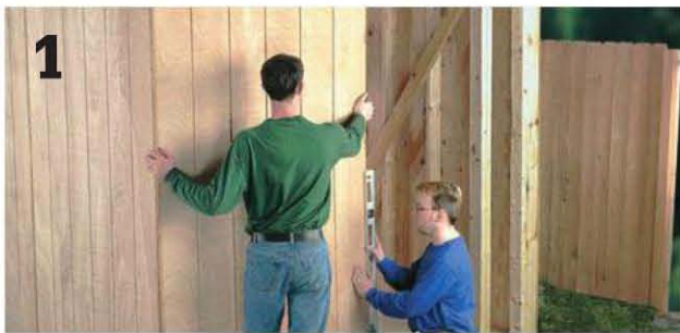
1 Install the plywood siding vertically. Plumb each sheet and fasten it to the framing with 6d nails.
