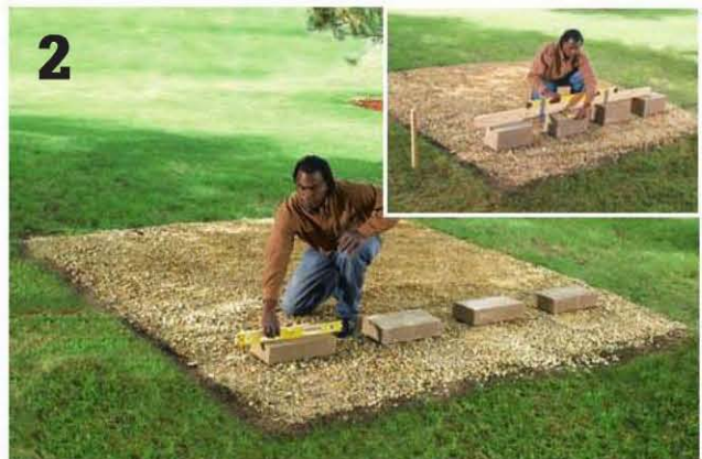
Set a block at the highest point on the site , check it with a level, and adjust as needed. (Inset) Use a level and board spanning across the blocks to establish the height of each stack so all the tops are level.
