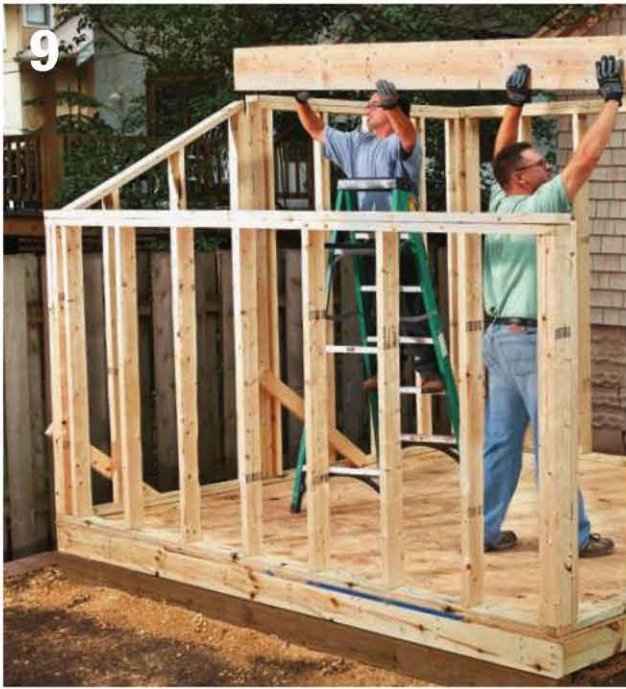
9 Set the main header on top of the sidewall posts and toenail it in place with 16d common nails. The main header ends should be flush with the outsides of the side walls.
