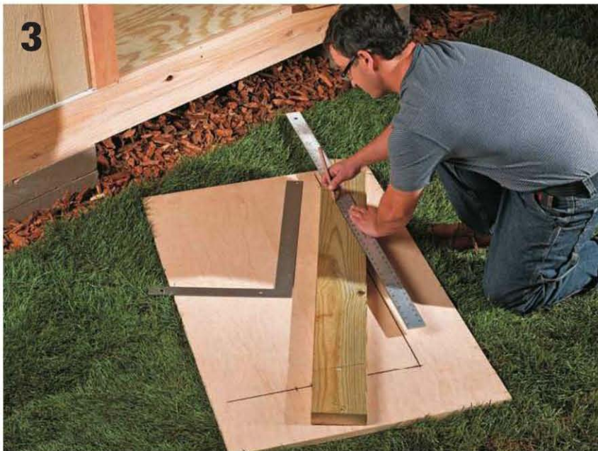
Use perpendicular layout lines to mark the angled end cuts on the first stringer.
