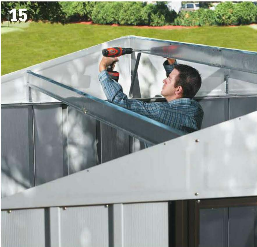
15 Drive fasteners to affix the roof beam to the gable ends and install any supplementary support hardware for the beam, such as gussets or angle braces.
