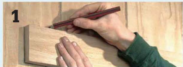
Trace along the trim to mark the cutting lines for removing the siding.
