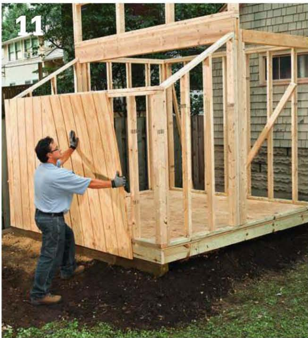
11 Install T1-11 siding on the front wall , starting at the left side (when facing the front of the shed). Cut the siding to length so it's flush with the top of the top plate and the bottom of the floor joists. Make sure any vertical seams fall at stud locations. Add strips of siding to cover the framing on the clerestory wall. Install siding on the rear wall, starting at the left side (when facing the rear side of the shed).
