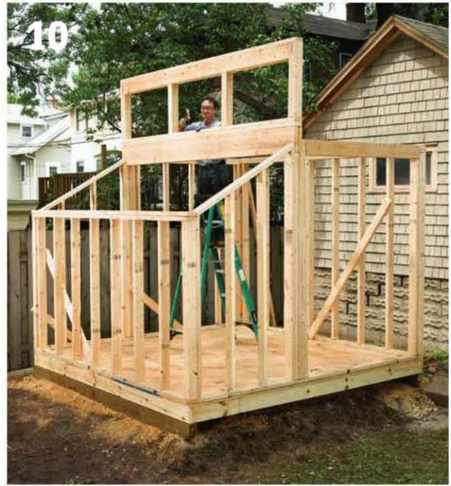
10 Lift the clerestory wall frame onto the main header. Orient the wall so it is flush in front and on the ends and then attach it to the main header with 16d nails.
