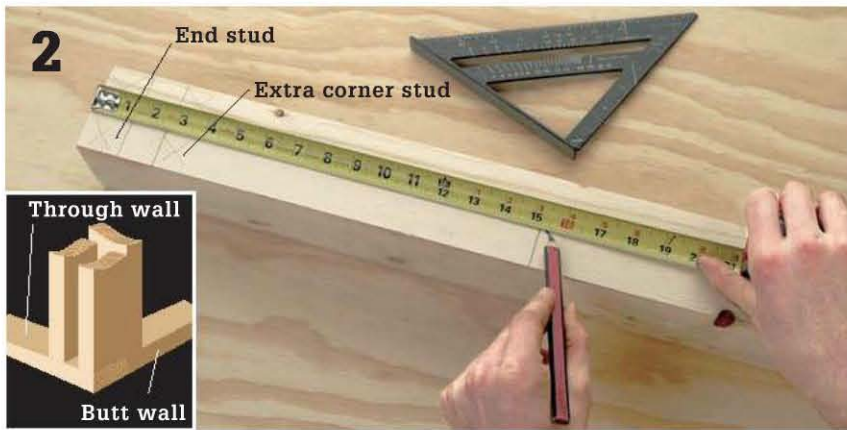
2 Mark the stud layout onto the wall plates, designating the stud locations with Xs. Through walls have an extra corner stud 2\frac{3}{4} " from each end.
