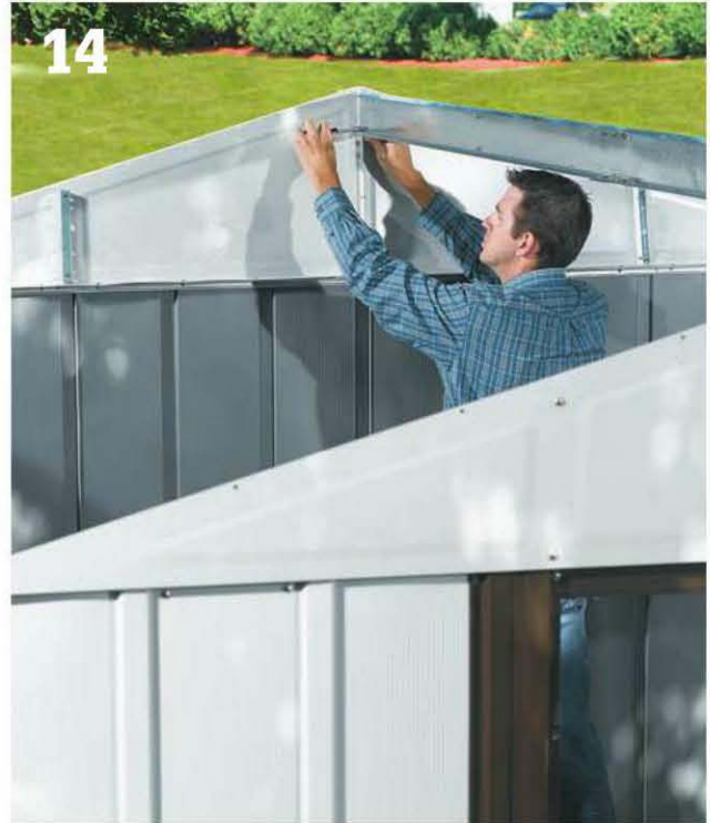
14 Fit the main roof beam into the clips or other fittings on the gable panels. Have a helper hold the free end of the beam. Position the beam and secure it to both gable ends before attaching it.
