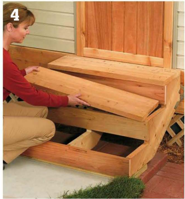
Trim the rear tread boards as needed to fit behind the front treads.
