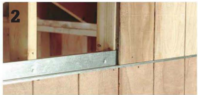
2 Add galvanized metal flashing between rows of siding to prevent water from entering the seam.
