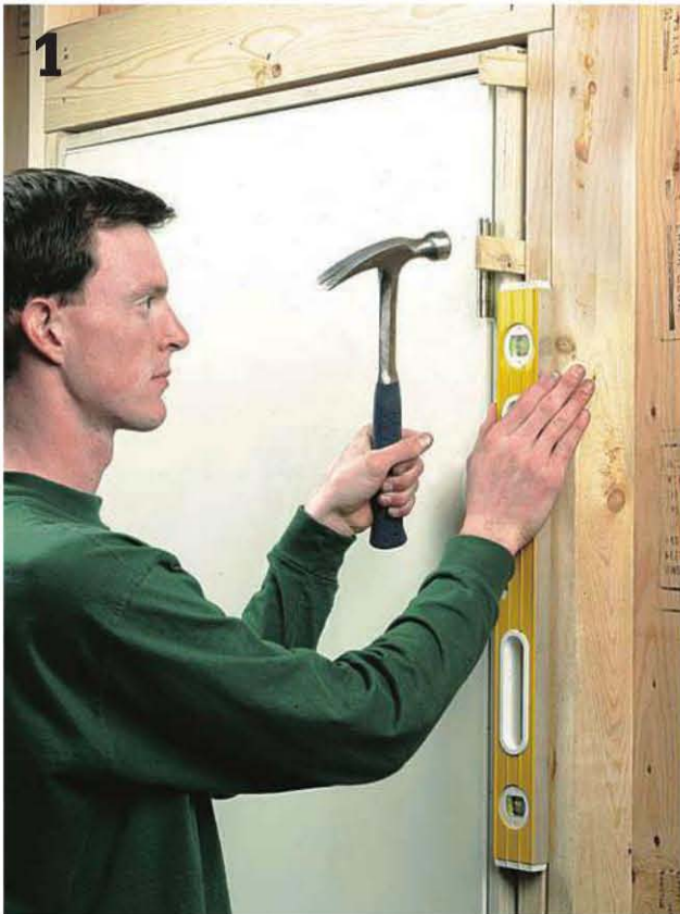
Plumb the door jamb , working from the top down. Fasten through the jamb and each shim pair with a casing nail.
