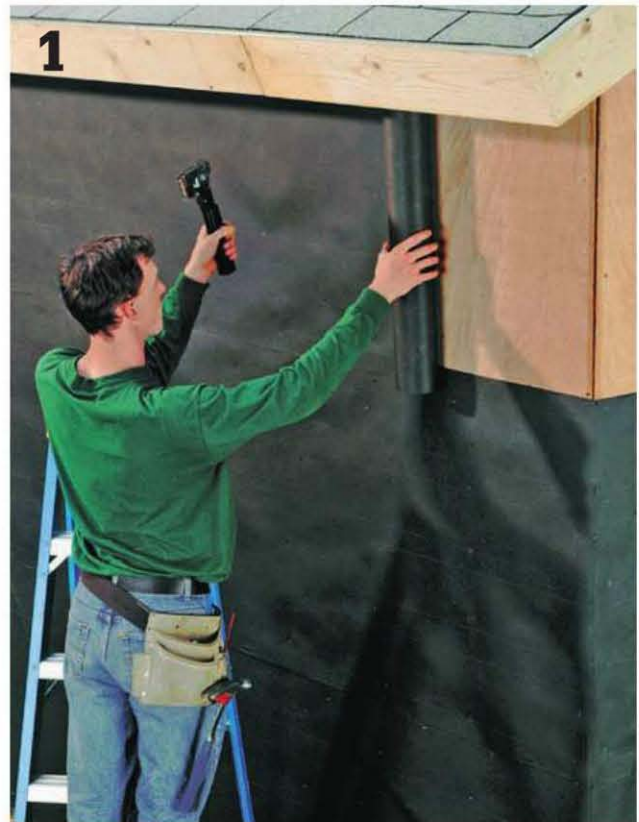
Install plywood sheathing over the entire frame, then staple building paper over the sheathing.
