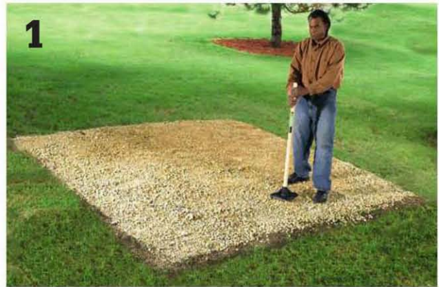
Create a bed of compacted gravel centered at each block location in your layout.
