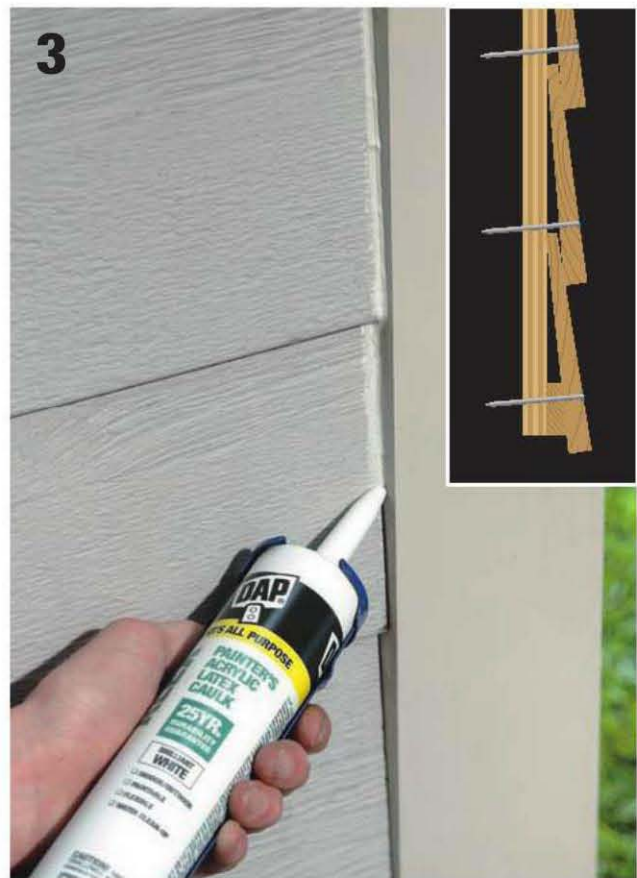
Drive siding nails into the studs, just above the preceding course (inset). Caulk all end joints after the installation.
