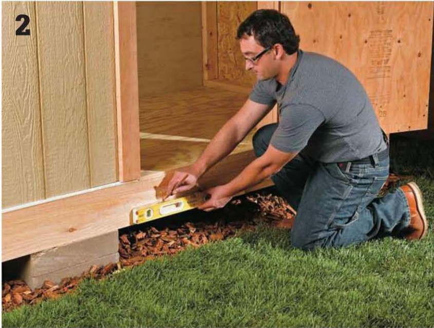
Mark a level line 4\frac{5}{8} " below the floor to locate the top edge of the ledger.
