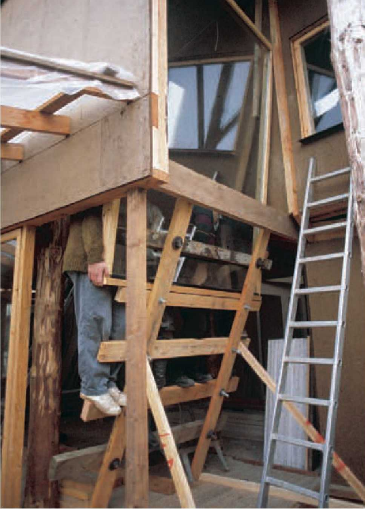
Four strong people lift a large double-glazed window to a high level up a purpose-made 'ladder'.
