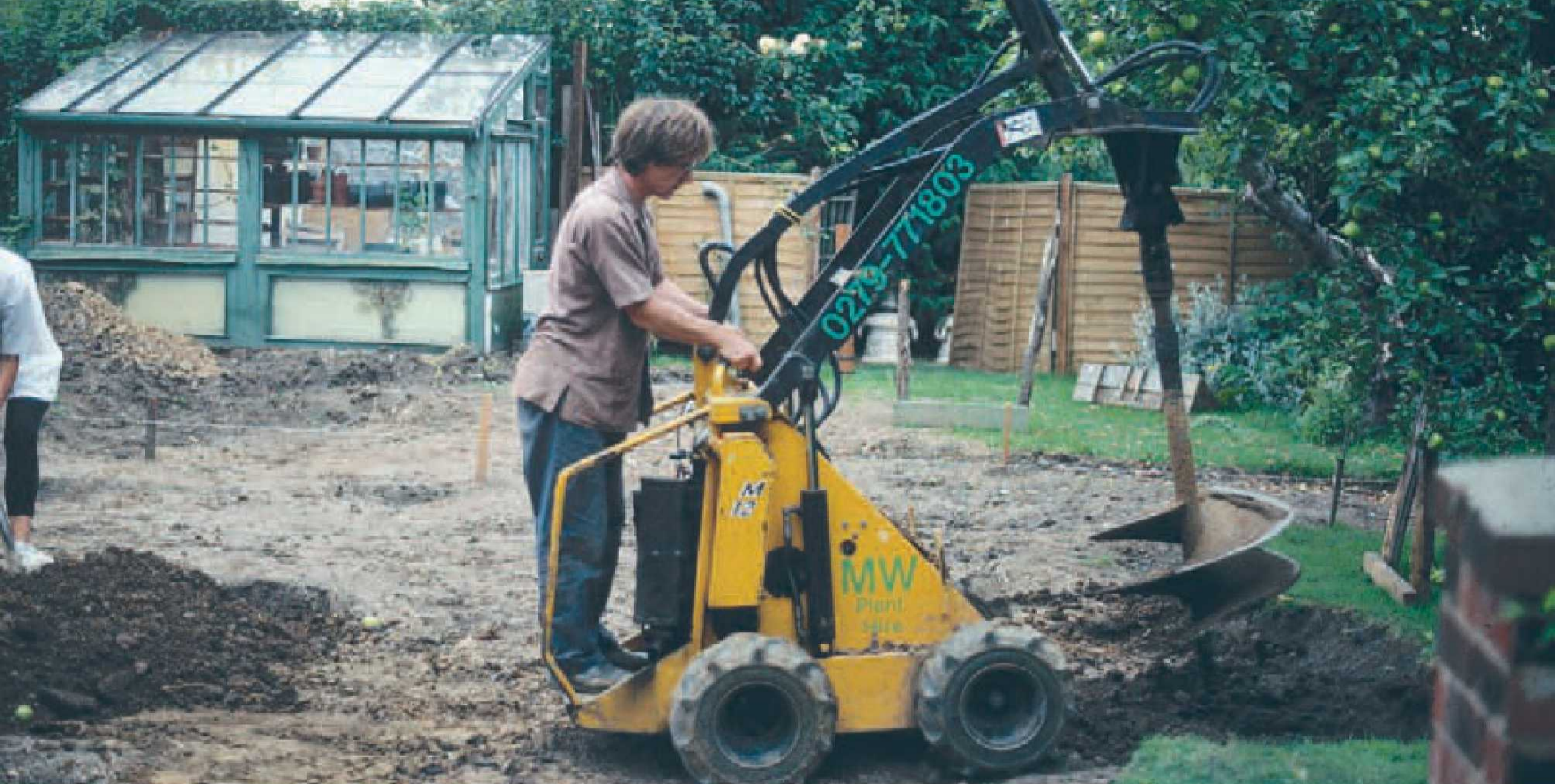
Foundation pads are excavated by a machine designed for drilling holes for fence posts.
