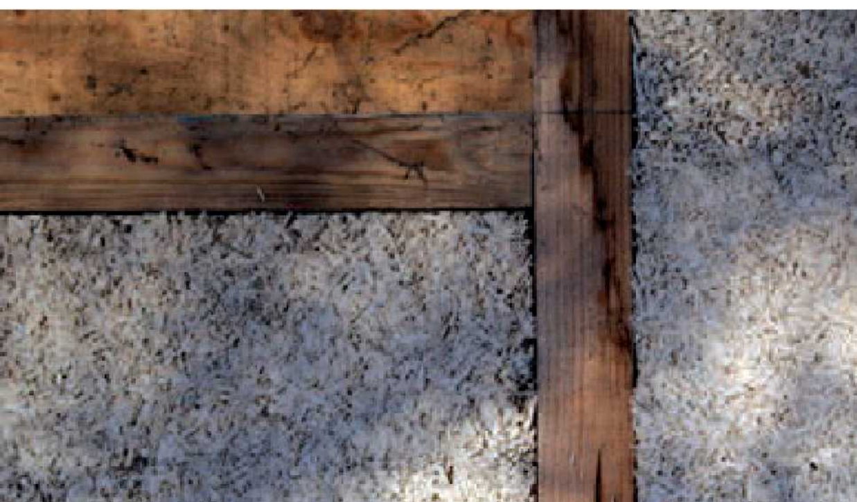
A wall of a hemp and lime mix within a timber frame.
