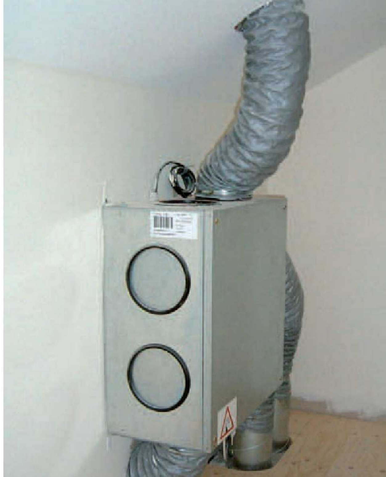
The principal source of heat loss in a well insulated airtight home is ventilation – this heat recovery system extracts up to 90% of the heat from stale air and uses it to pre-heat incoming fresh air.
