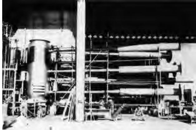
Photo of the “Mike” Device During Construction. The Actual Device is the vertical cylindrical structure on the left. The horizontal pipes leading from the device to the right are the pipes for measuring radiation emissions that would allow scientists and engineers to determine if each stage fired, and if so, how efficient the reaction was.
