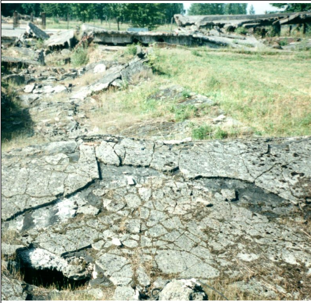
Illustration 15: The collapsed reinforced concrete roof of morgue #1 of Krema II at Birkenau in August 2000.
