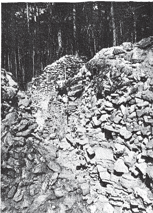
Fig. 5 Current profile of the crumbling wall
