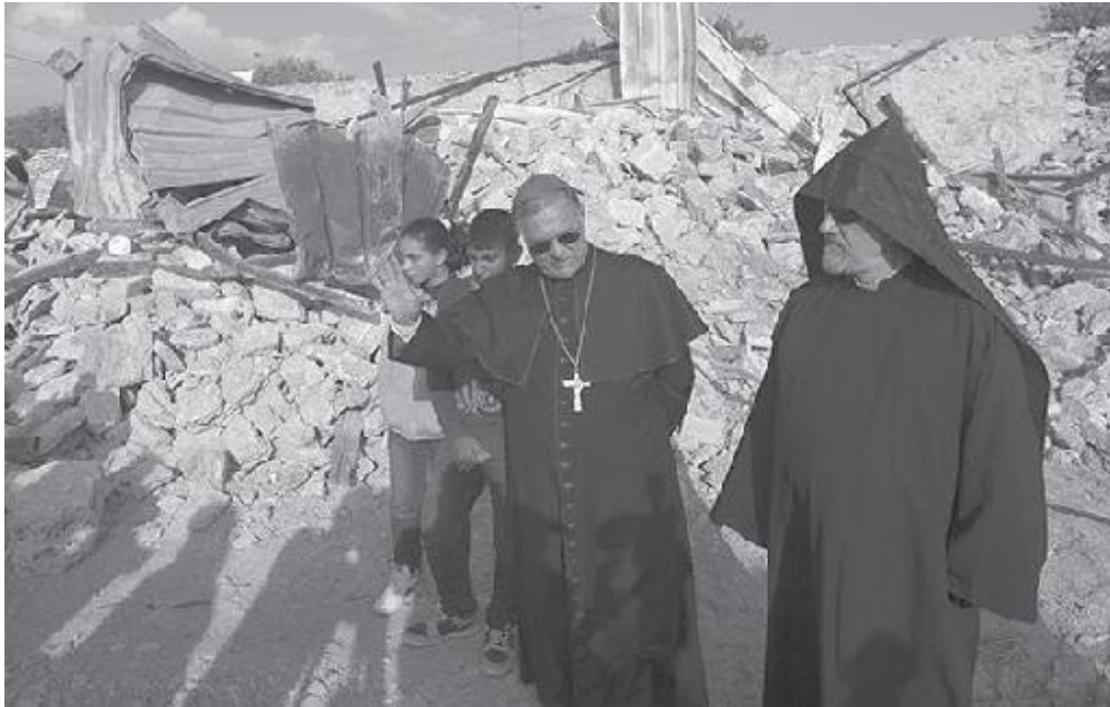
Monsignor William Hanna Shomali, Auxiliary Bishop of Jerusalem, surveys the demolition of a house owned by the Latin Patriarchate of Jerusalem.
