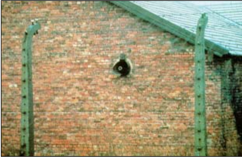
Fig. 19: Ventilation outlets from the disinfestation wing of building BW 5b, without equipment today. The ends of the water pipes are visible inside; see also Fig. 20.
