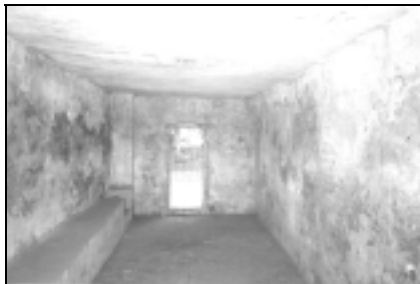
Fig. 65: Zyklon B disinfestation chamber in Stutthof camp, interior view taken from the south door. (© Carlo Mattogno 318 )
