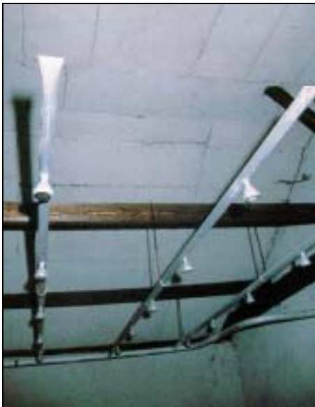
Fig. 20: Water pipe system with shower heads in the disinfestation wing of building BW 5b. These water pipes have no connection; they terminate in the ventilation outlets. See Fig. 19.
