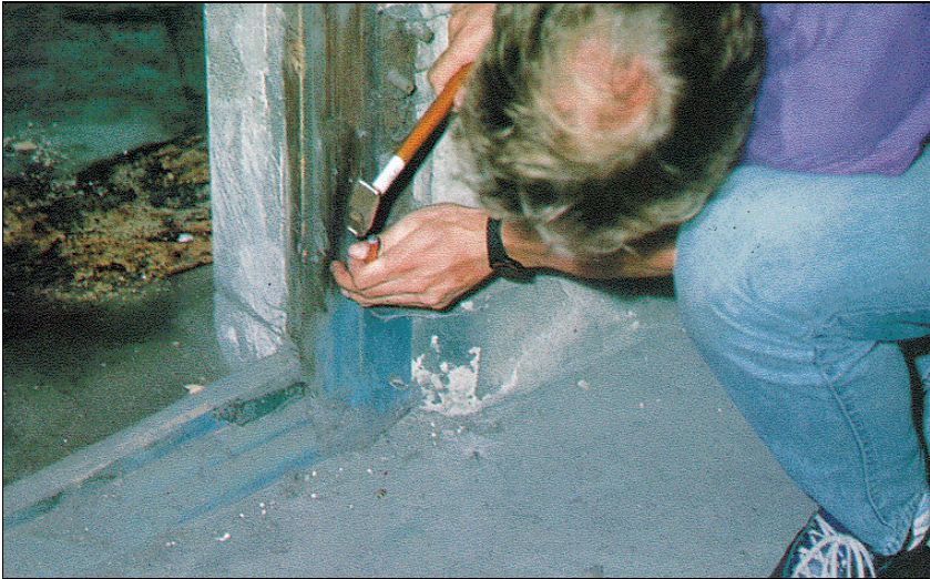
Fig. 70: Picture of the door frame in disinfestation wing of building 5a. the lower, rusty hinge has developed Iron Blue under the influence of hydrogen cyanide. Sample taking location of sample no. 18.
