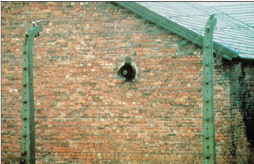
Fig. 20: Ventilation outlets from the disinfestation wing of building BW 5b, without equipment today. The ends of the water pipes are visible inside; see also Fig. 21.
