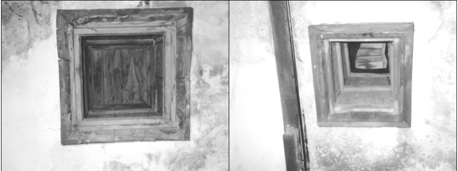
Illustration 5: and Illustration 6: Eastern (top) and western (right) opening in the ceiling of the delousing facility in hut 41, concentration camp Majdanek (cf. map, illustration 1). © C. Mattogno
