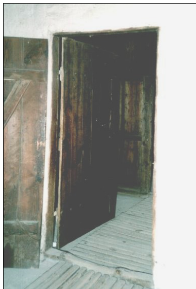
Photograph XVII: Barrack 41, gas chamber, north door. The inside of the door is marked by the typical discolorations that are also visible on the outside of the south door (Photograph XVIa); hooks for the latches are missing from the door frame, unlike on the frame of the south door (Photograph XVI). © Carlo Mattogno
