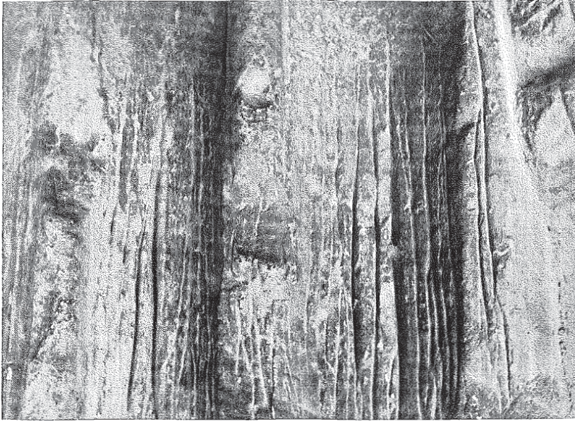
Fig. 2 Frankfurt a. d. Oder Cathedral. Wetzrillen to the left of the north-facing door to the baptismal chapel
