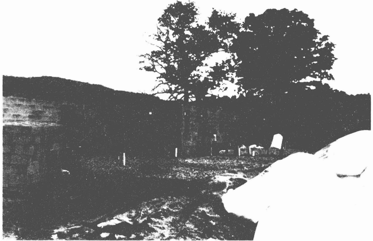
The School for Gifted Boys under construction. The walls are of 8" CBS. This picture shows part of
