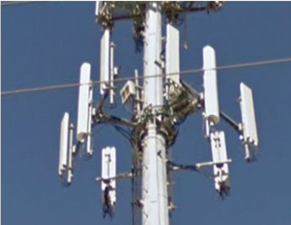
Figure 3. Note the box enclosure with vents in the center of this image. This is an AT&T equipment tower, owned by Crown Castle.
