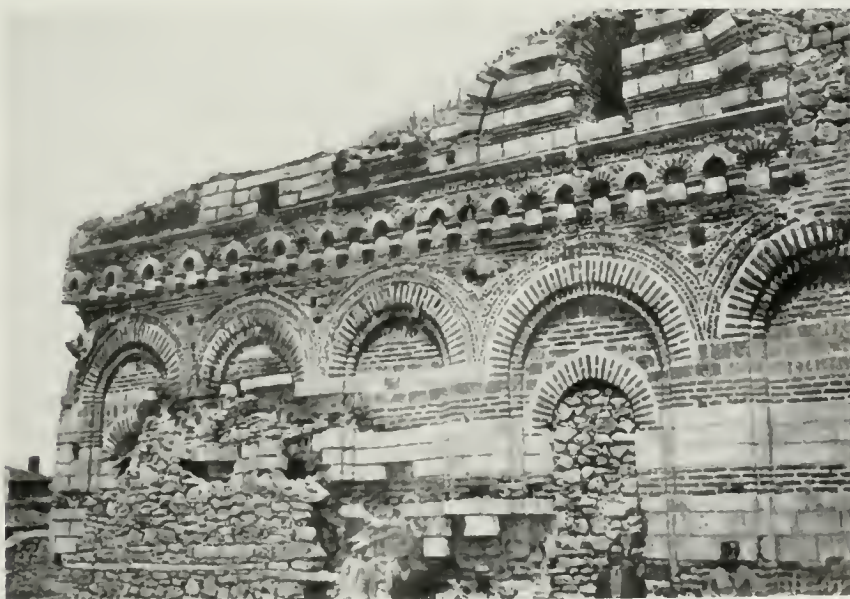
Fig. 20. — The church of St. John at the harbour in Mesembria, south front; 14 th cent. Before the destruction by the earthquake of 1913.
